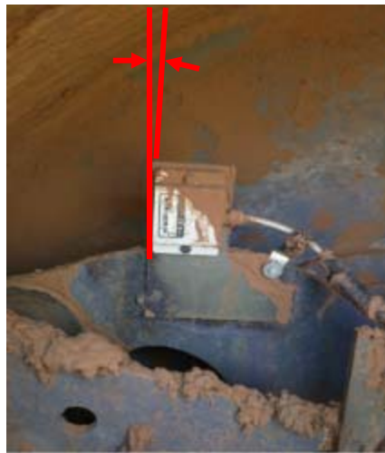
Figure 5.1 – Non-Vertical Mounting of Retrofit Accelerometer.
