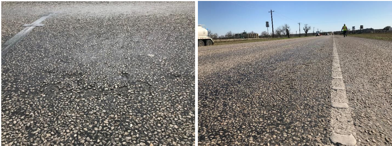
Figure A.7. Raveling and Rutting in SH 16-Atascosa County
