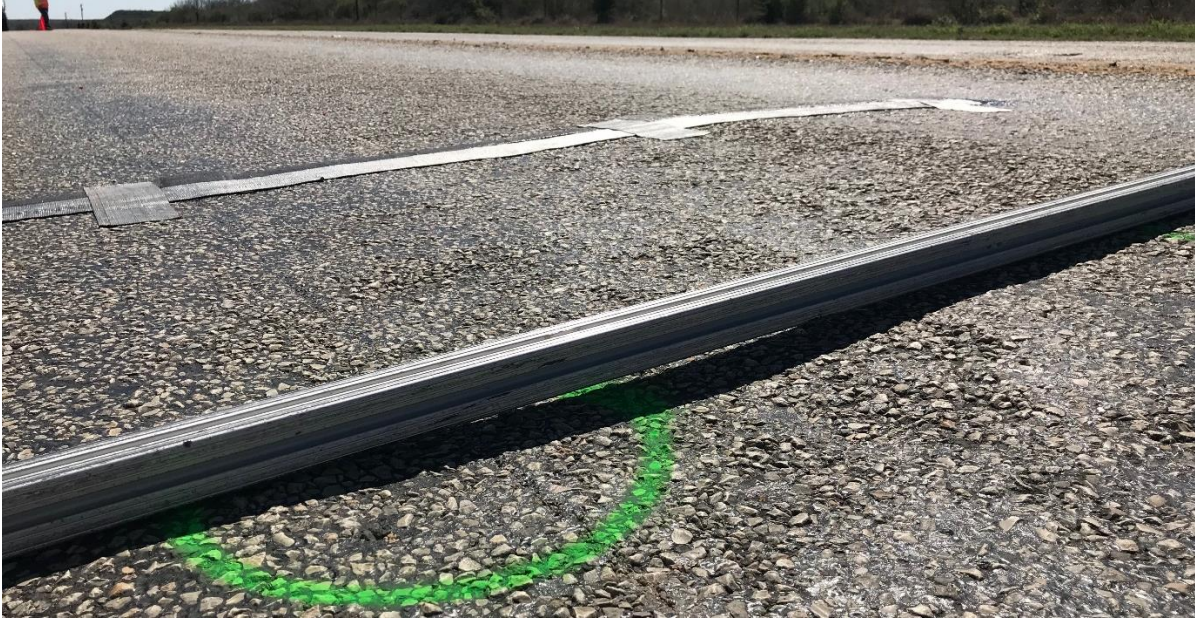
Figure A.10. Rutting and Flushing in FM 624 - McMullen County
