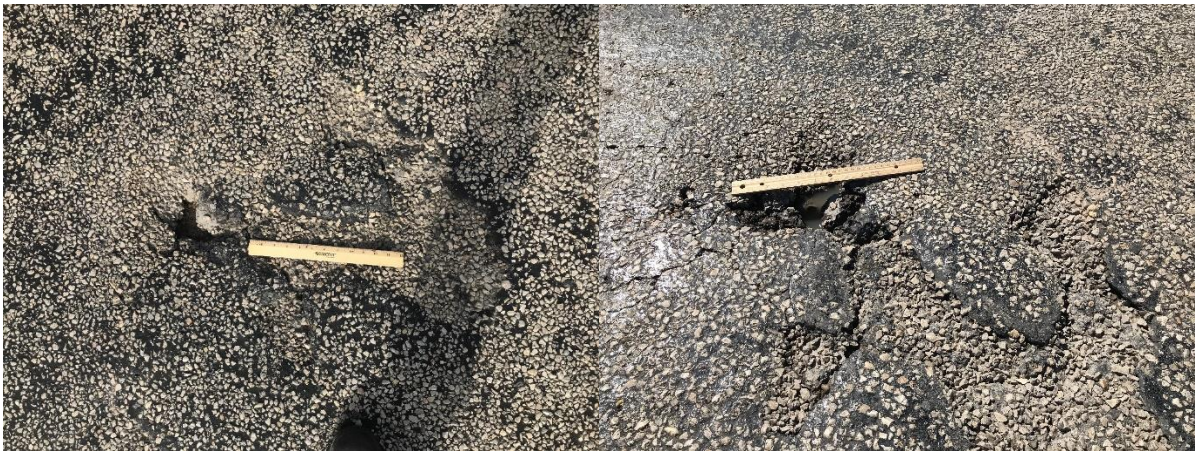
Figure A.11. Pothole Formation in FM 624 - McMullen County
