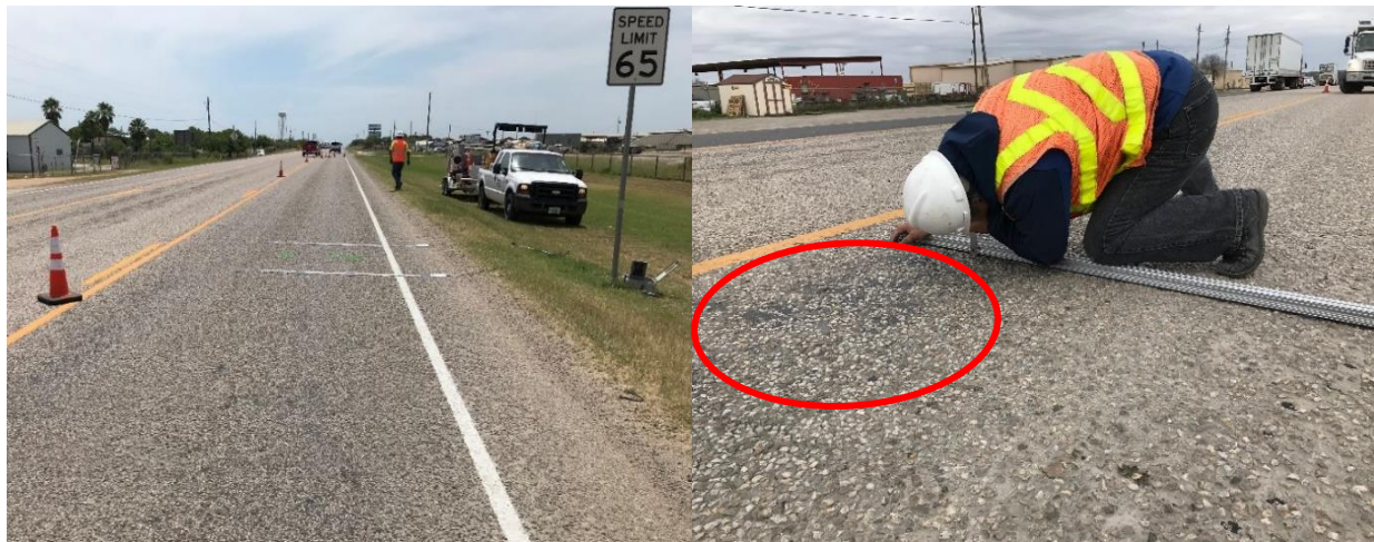
Figure A.5. Flushing and Shallow Rutting in US 83 -Dimmit County
