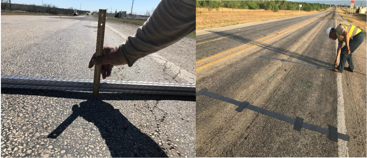
Figure A.8. Rutting and Flushing in FM 99 - McMullen County
