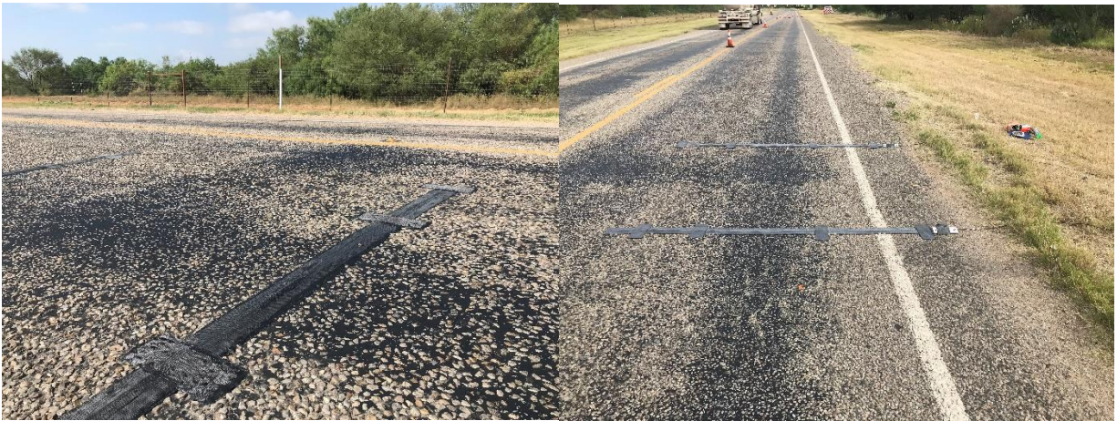
Figure A.1. Severe Flushing in FM 468 - La Salle County
