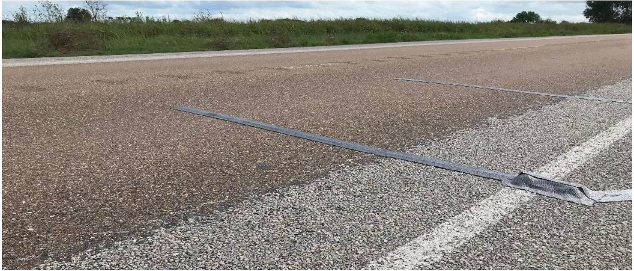
Figure A.18. Pavement Conditions of SH 119 - Dewitt County
