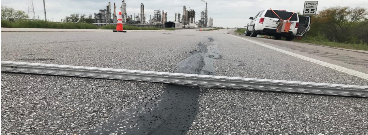
Figure A.12. Rutting in US 281 – Live Oak County
