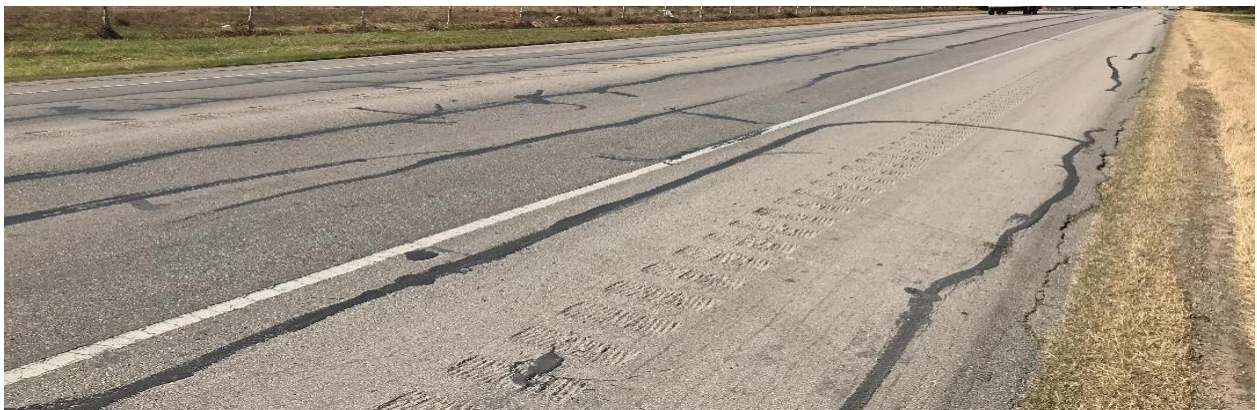
Figure A.19. Pavement Conditions of US 183 - Gonzales County
