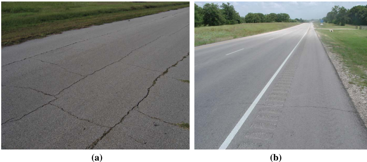
Figure 2-3: (a) Block Cracking and (b) Transverse Cracking in HMA with Stabilized Base Materials (Sebesta and Scullion 2004).
