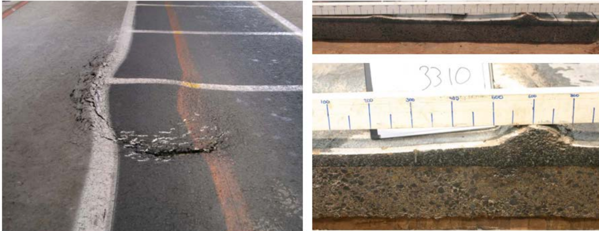
Figure 2-1: Rutting of the HMA Layers without Deformation of the Cemented Base Layer (Austroads, 2008).
