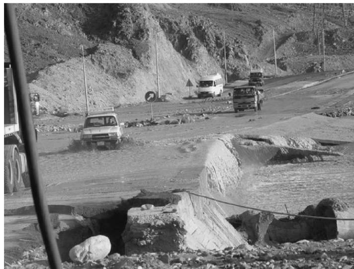
Figure B.25 Flash flood damage to highways crossing a stream in the Wadi Watir Sinai catchment, Egypt (Kotb and El Belasy, 2007)
