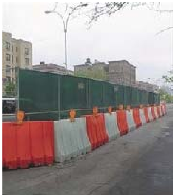
Longitudinal Channelizing Devices (LCDs)
