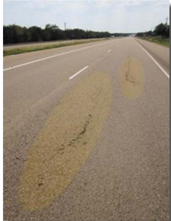
Figure 1. Cyclical Cracking on a Roadway.
