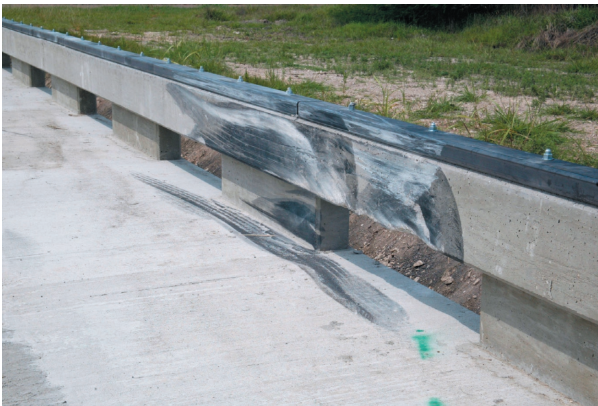
After-test photo of bridge rail showing marks from vehicle. Note that tire contacted post.
