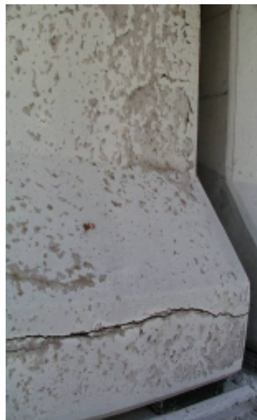
Figure 1: Example of field damage from Premature Concrete Degradation (PCD)
