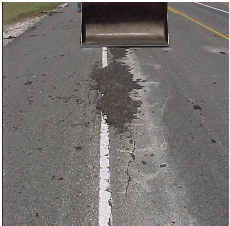
Figure 1. Premature Cracking Associated with Damaged Underseal.
