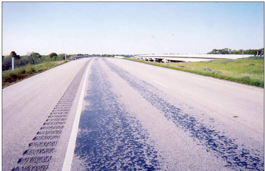
Figure 2. Underseal Bleeding through the Asphalt Concrete Overlay.
