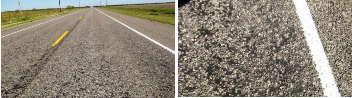
Figure 11. Example of Inadequate Performance on 16-CRP-2 after the First Winter.
