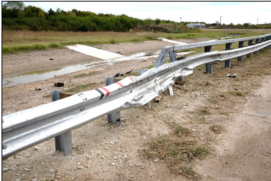
Figure 7.5. Transition at the Impact Location after Test 441203-01-2.
