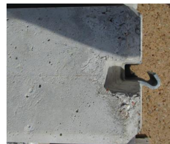
(c) Joint (JJ-Hook) Deformation
