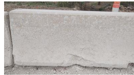
(a) Concrete Spall
