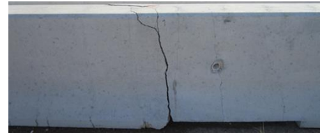
(b) Segment Crack
