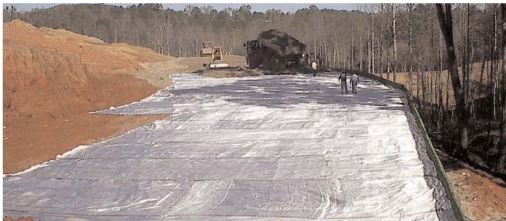
Above: The HS400PP and HS800PP high strength geotextiles were embedded between 4.5-6m (15-20ft) in length.
