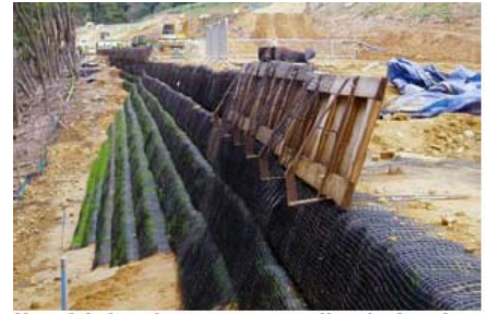
Use of timber shutter system to align the face for the steep reinforced slope sections
