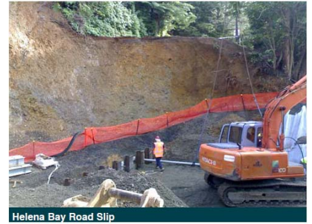
Helena Bay Road Slip
