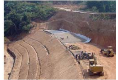
Installation of the drainage blanket at the base of the reinforced slope
