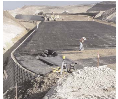
The contractor was able to install 5,000 yds 2 of Miragrid® geogrids a day.
