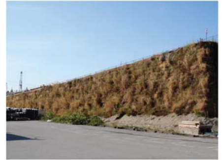
Nearly two dozen Sierra Slopes were installed as part of the Port Mann Bridge Project. The bridge will double existing lanes from five to ten and will sustain Vancouver's traffic growth over the next two decades.
