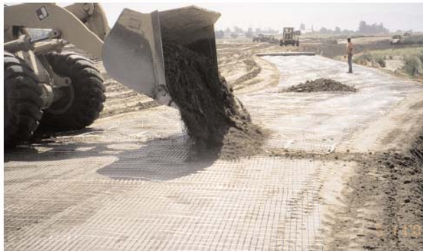
Enkagrid® PRO is placed in 3 foot intervals for a total slope of 20 feet.
