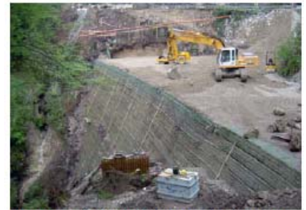
Steel mesh facing used to form a smooth slope face which aids in vegetation growth and aesthetics
