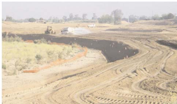
Enkagrid PRO was used to stabilize the slope under the water level.
