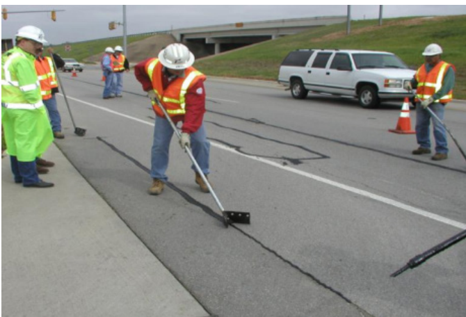
Figure 1. Premature Cracking in New Overlays.
