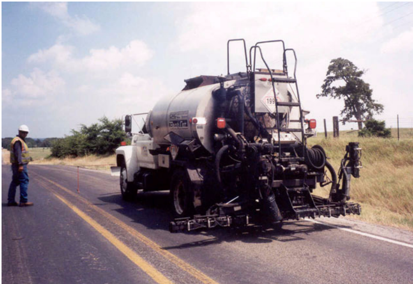
Figure 7-11. Typical Distributor Spray Bar.
