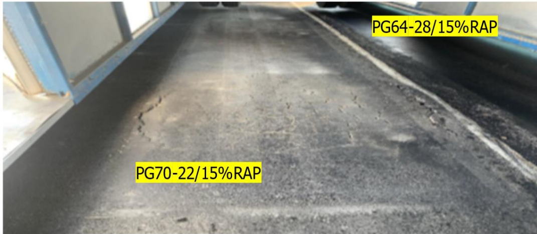
Figure 59. Fatigue Cracking on Test Section O with PG70-22 (Left) and Section P with PG64-28 (Right).
