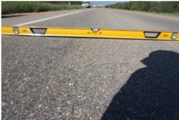
Rutting in Outer Wheel Path: 1/16–8/16 in. 10/09/2017
