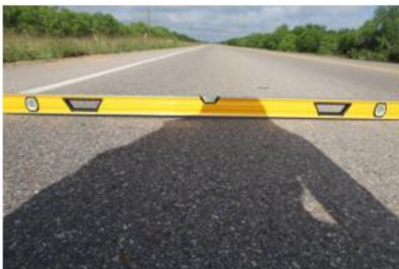
Rutting in Outer Wheel Path: 1/16–8/16 in. 03/29/2018
