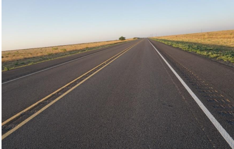
Figure 52. No Cracking on the Test Section with PG64-34 on SH 214.
