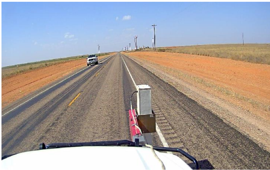
Figure 46. Pavement Condition of SH 214.
