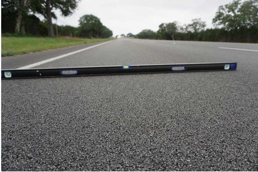
Figure 71. No Rutting on the Test Section with PG70-28 on SH 71.
