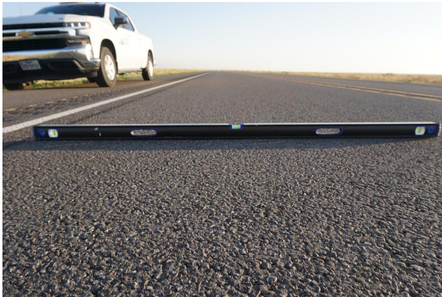
Figure 51. No Rutting on the Test Section with PG64-34 on SH 214.
