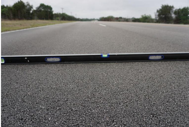
Figure 73. No Rutting on the Test Section with PG70-22 on SH 71.
