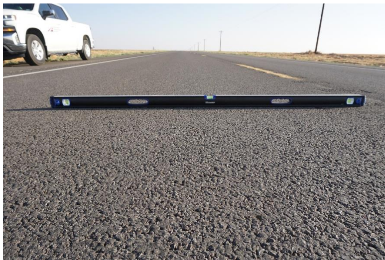
Figure 53. No Rutting on the Test Section with PG70-28 on SH 214.
