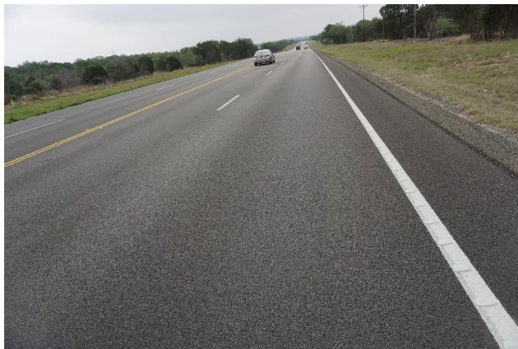
Figure 74. No Cracking on the Test Section with PG70-22 on SH 71.
