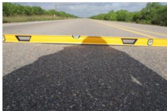
Rutting in Inner Wheel Path: 1/16–8/16 in. 03/29/2018
