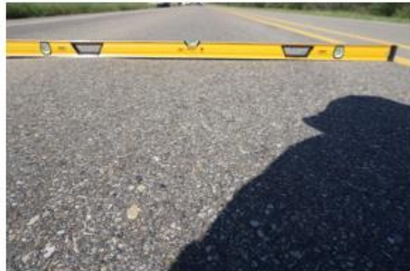
Rutting in Inner Wheel Path: 1/16–8/16 in. 10/09/2017
