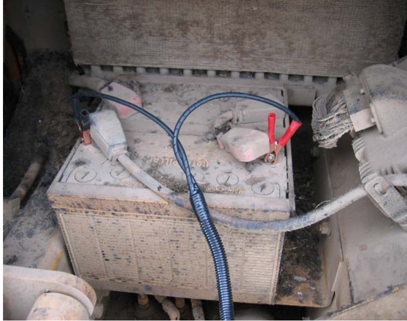
Figure 7. Master Power Cable Connected to Paver Battery.
