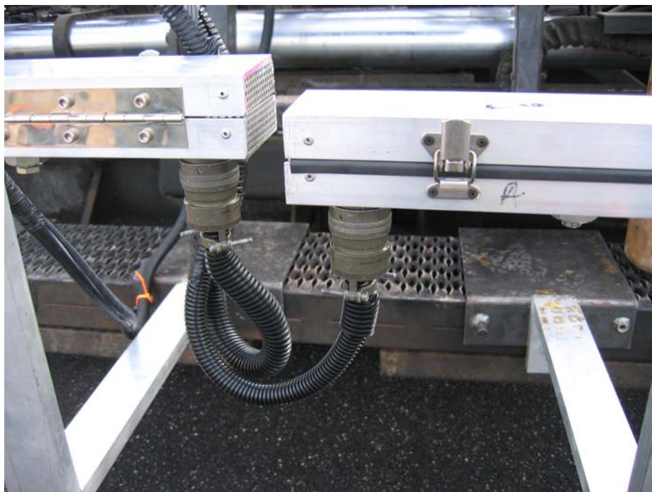
Figure 4. Master Control Cable Connected to IR Bars.
