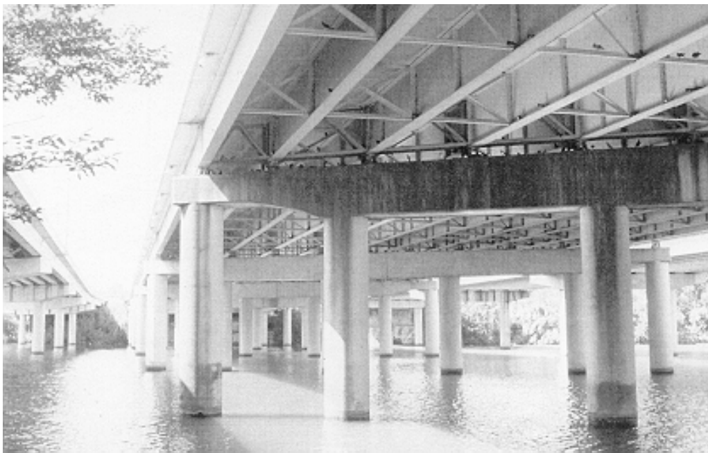
Figure 4-7: View of diaphragm framing of northbound structure looking south from the north shore of Town Lake.
