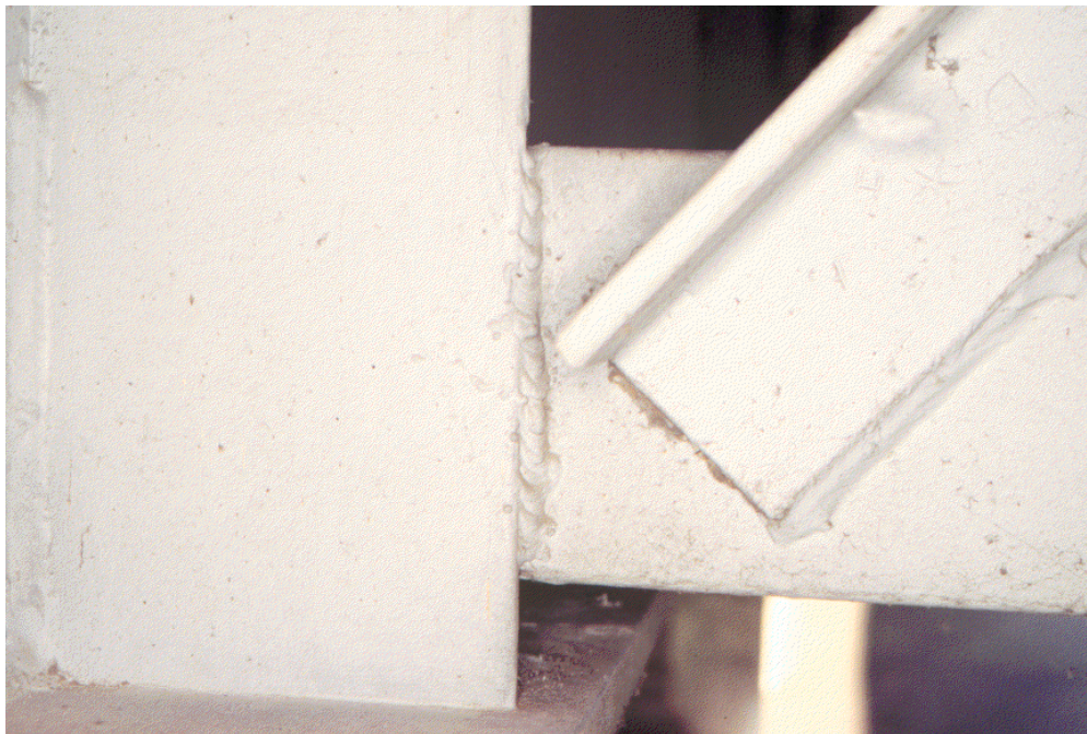
Figure 4-9: View of cracked fillet weld at diaphragm connection, Town Lake Bridge.
