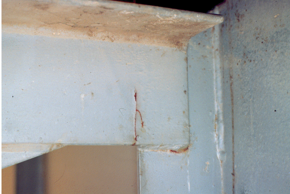
Figure 1-9: Fatigue crack in cross frame upper strut at diagonal connection.
