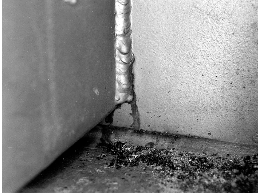
Figure 1-6: Fatigue crack at end of unstiffened web gap of cut-short termination detail.
