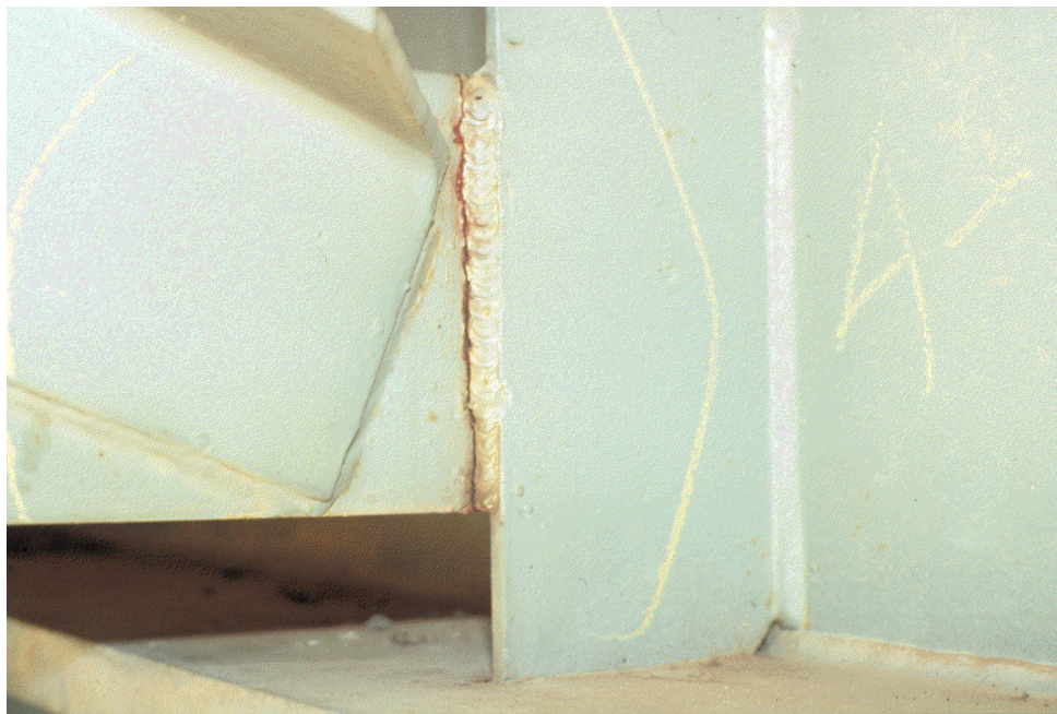
Figure 1-8: Fatigue crack in fillet weld between cross frame diaphragm lower strut and connection plate.
