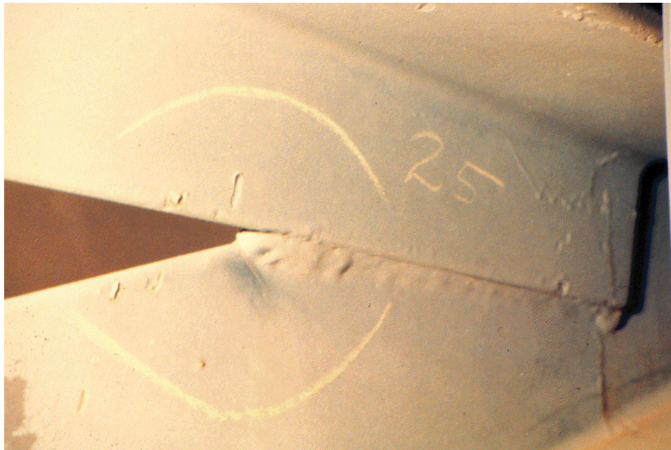
Figure 1-10: Fatigue crack in cross frame lower strut at diagonal connection.
