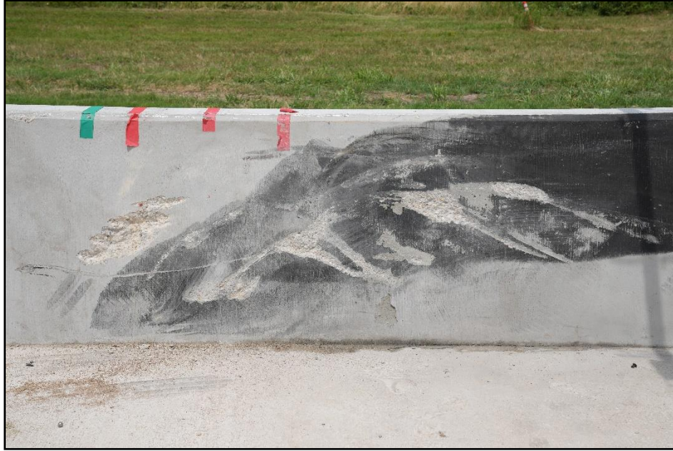
Figure 5.5. Perpendicular View of Luminaire Pole behind Single Slope Traffic Rail at Impact Location after Test 440863-03-1.
