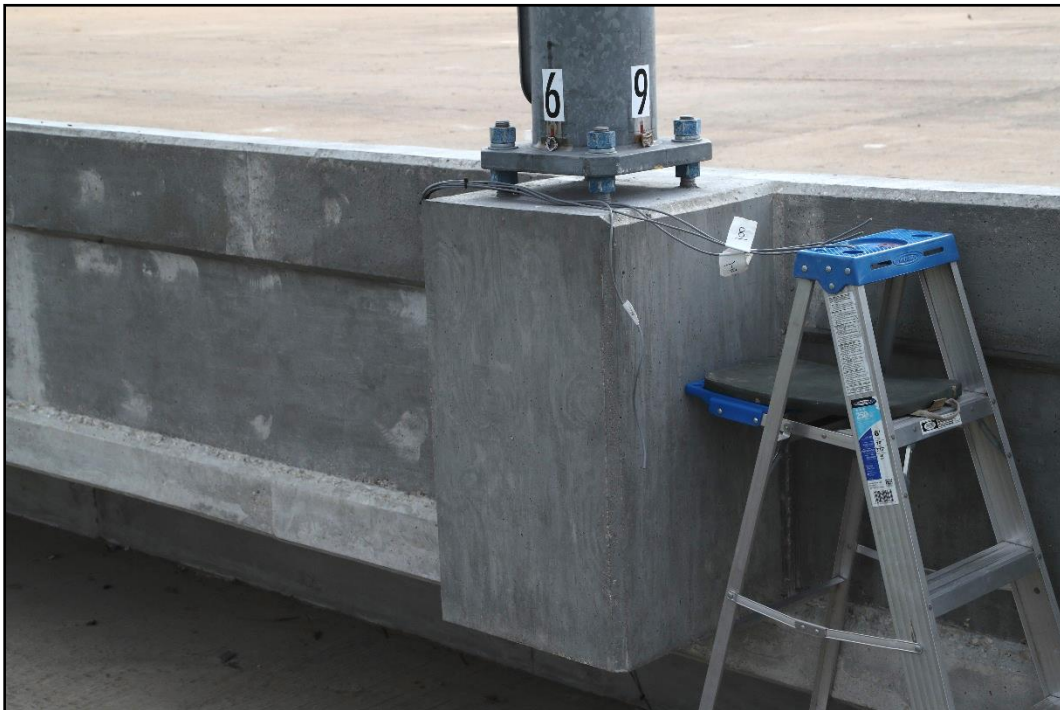
Figure 2.7. Field Side of the Luminaire Pole behind Single Slope Traffic Rail Prior to Testing.
