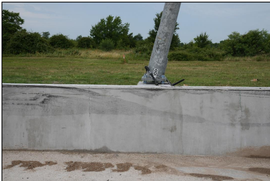
Figure 5.6. Traffic Side View of the Damage to the Base of the Luminaire Pole after Test 440863-03-1.
