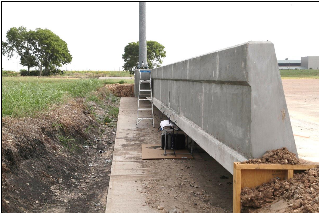
Figure 2.3. Field Side of Luminaire Pole behind Single Slope Traffic Rail Prior to Testing.
