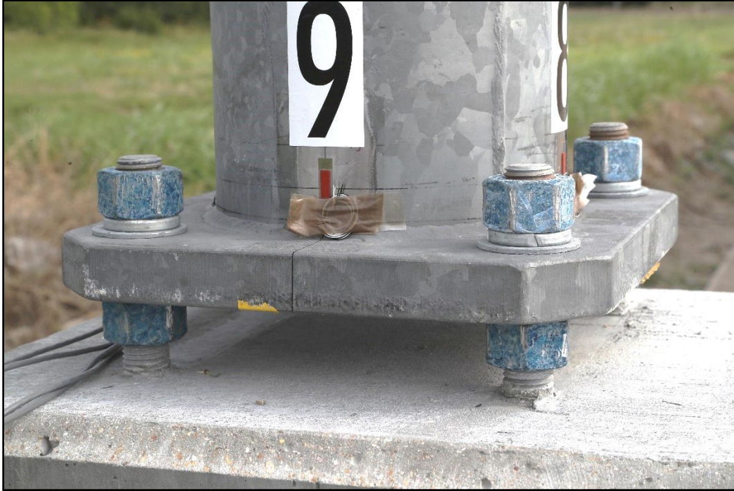
Figure 2.4. Base of the Luminaire Pole behind Single Slope Traffic Rail Prior to Testing.
