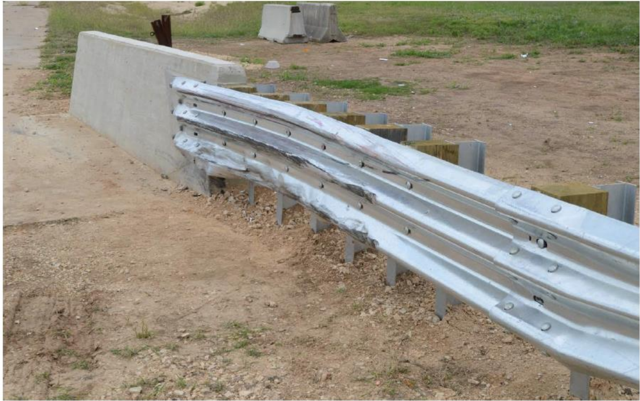
Figure 2.16. TxDOT TL-3 Transition after Testing (7).
