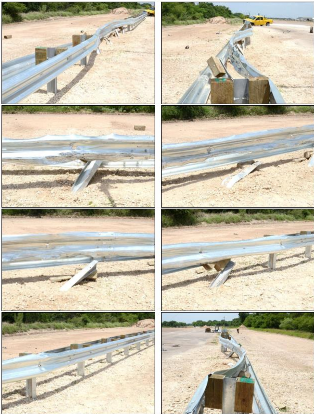
Figure 2.9. Installation after MASH Test 3-11 (Pickup Truck) (3).
