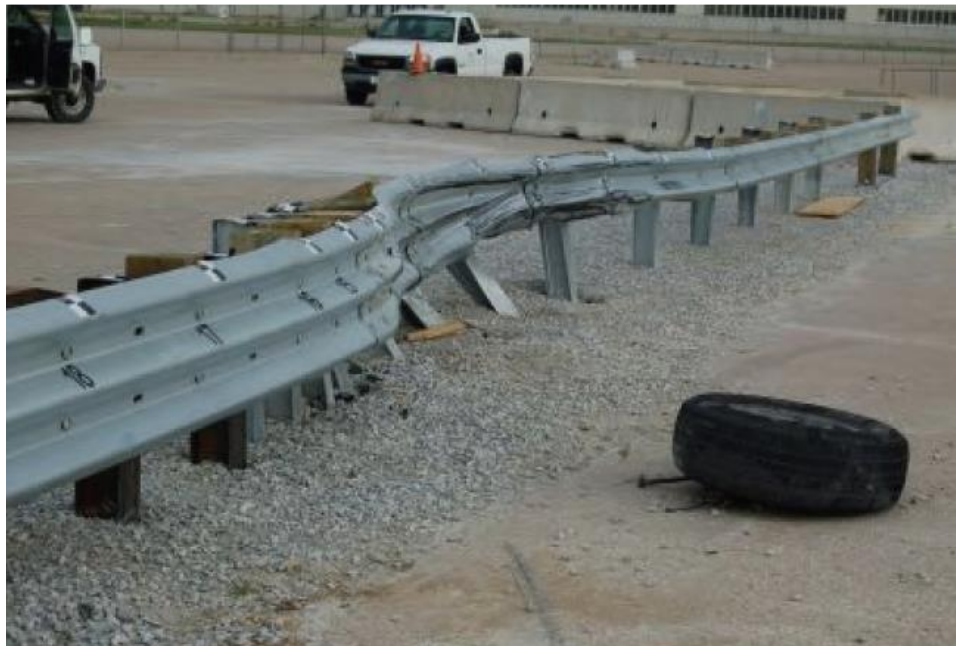
Figure 2.18. Rail Deformation after Testing (8).
