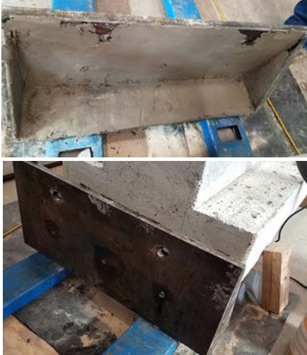
(a) Put grout on the anchor plate or channel and place the anchor plate or channel
