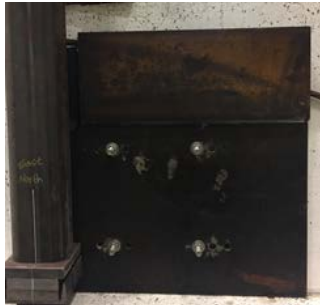
(c) Place side plate for the exterior test, mark and drill the holes, and install anchors
