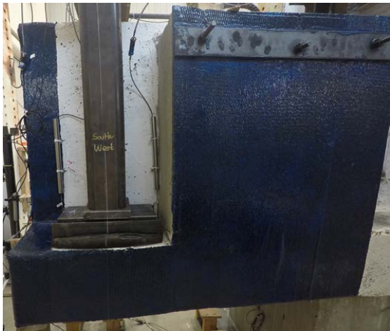
(c) North side at measured ultimate load
