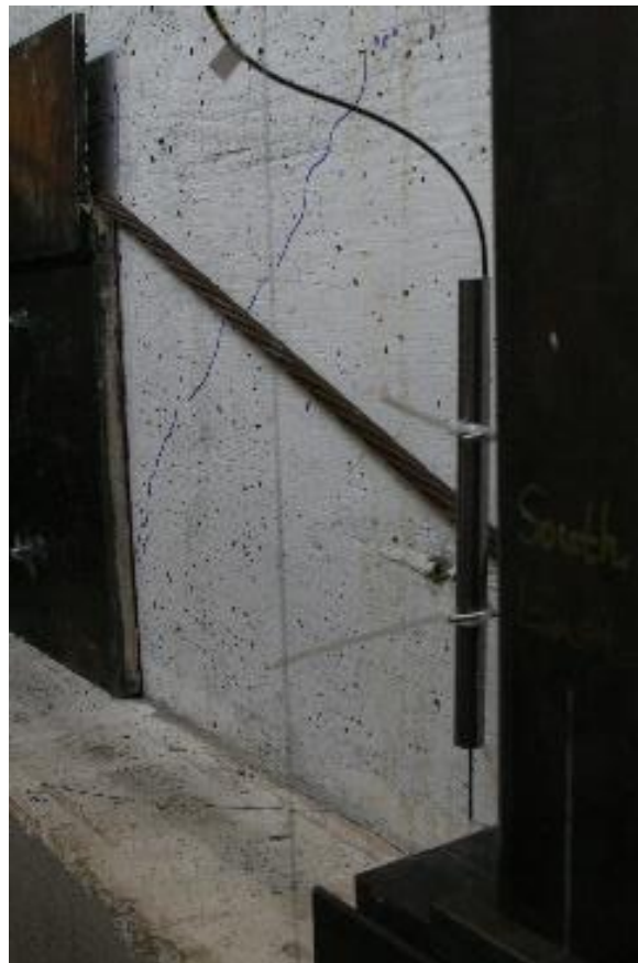
Figure 3.70. Observed Damage Before PT Jacking Operation.
