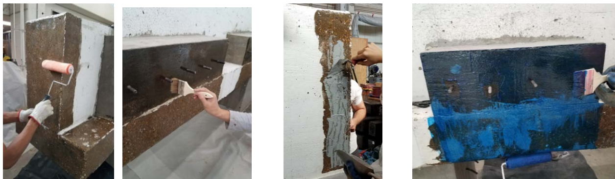
(a) Applying epoxy primer (b) Applying epoxy paste (c) Applying epoxy encapsulation resin
