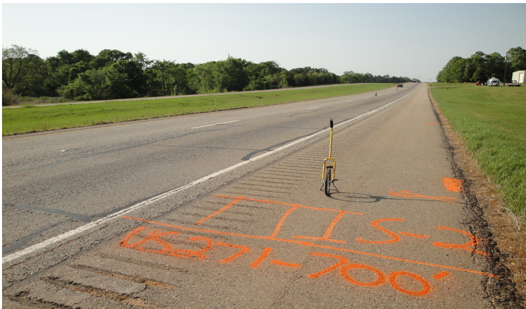
Figure 5-8. Reflective Cracking Observed in US 271 (Paris District).
