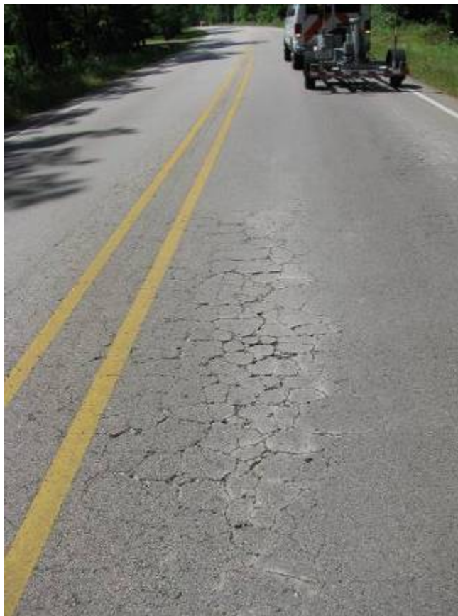
Figure 8. Alligator Cracking at South End of Project.
