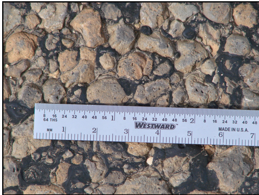
Figure 16. FM 503 Lightweight Grade 3 Seal Coat Texture.
