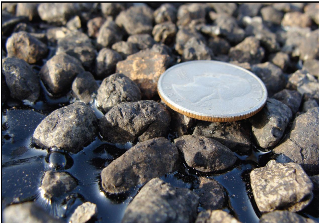
Figure 8. Proper Aggregate Embedment After Several Days of Traffic.
