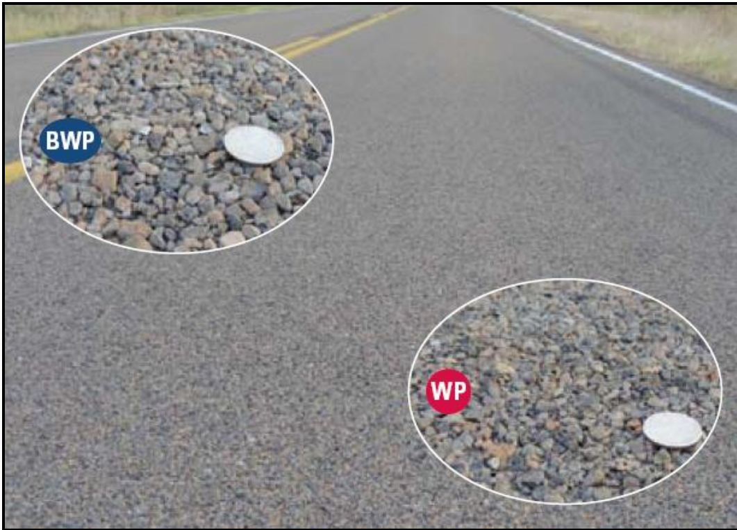
Figure 23. No Color Difference in Grade 4 Seal Coat.
