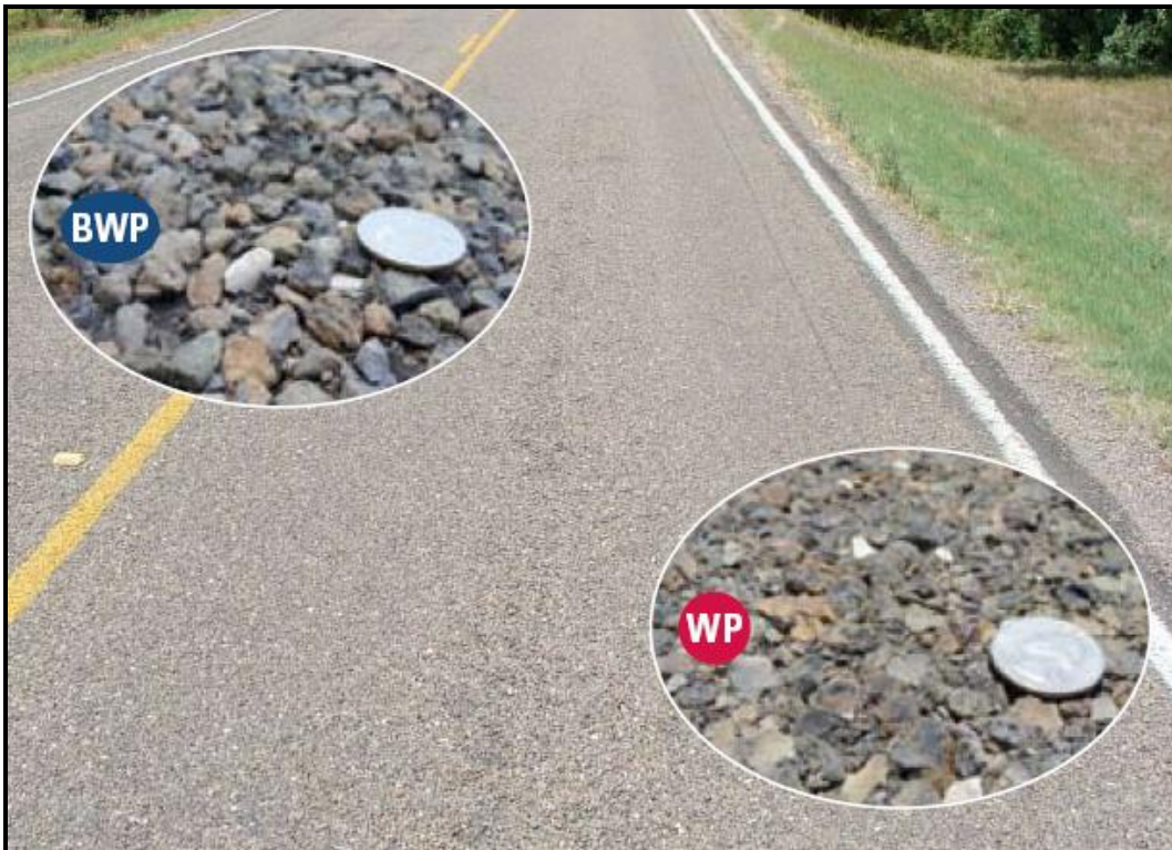
Figure 22. Slight Color Difference in Grade 4 Seal Coat.
