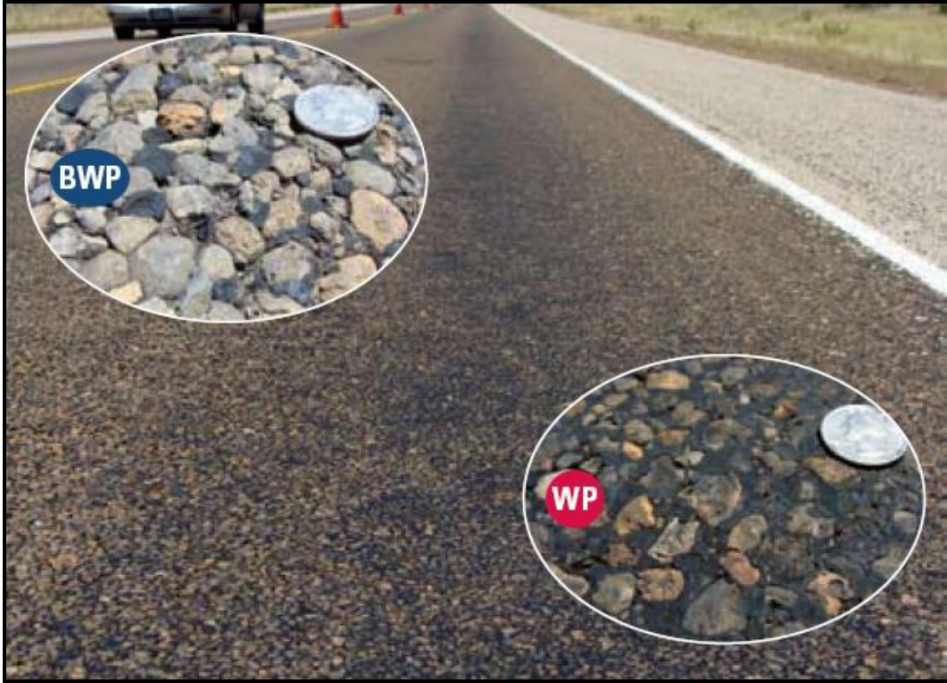
Figure 19. Moderate Flushing of Grade 3 Seal Coat.
