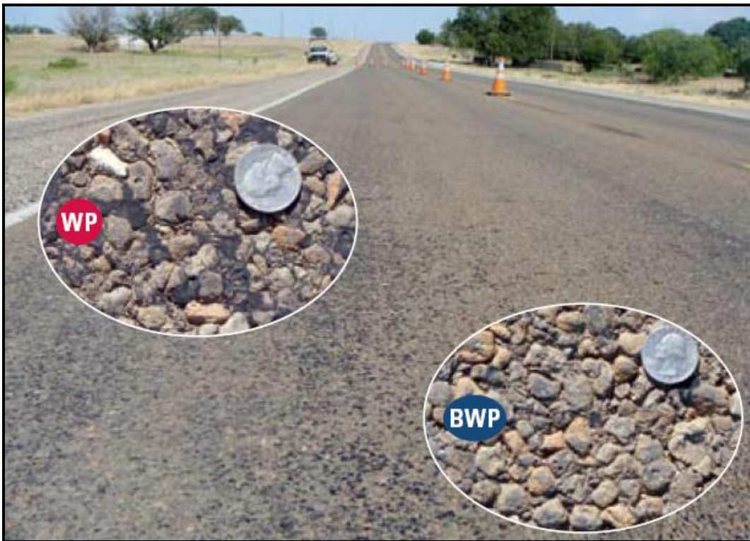
Figure 20. Mild to Moderate Flushing of Grade 3 Seal Coat.
