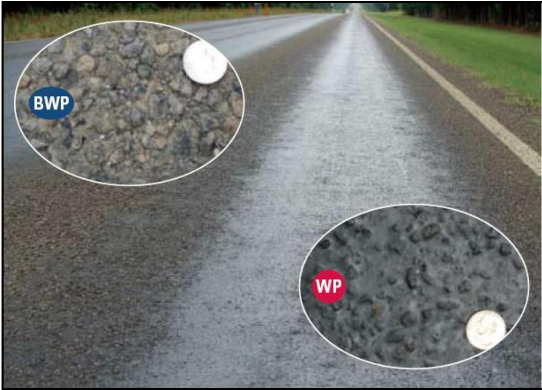
Figure 17. Severe Flushing of Grade 3 Seal Coat.
