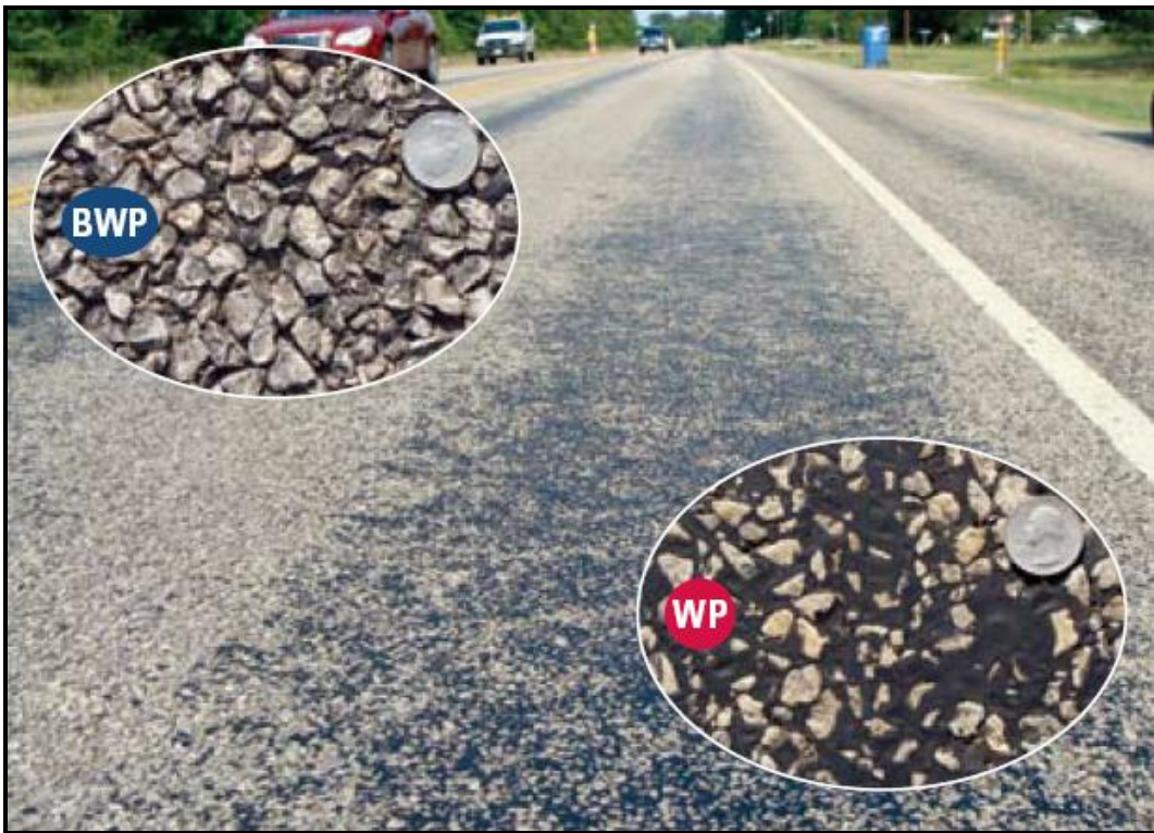
Figure 18. Moderate to Severe Flushing of Grade 3 Seal Coat.
