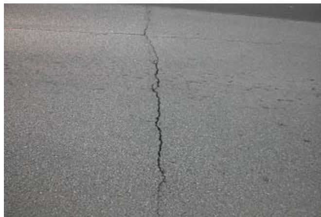
Figure 6-7. Example of Transverse Cracking on BU 59 (Lufkin).
