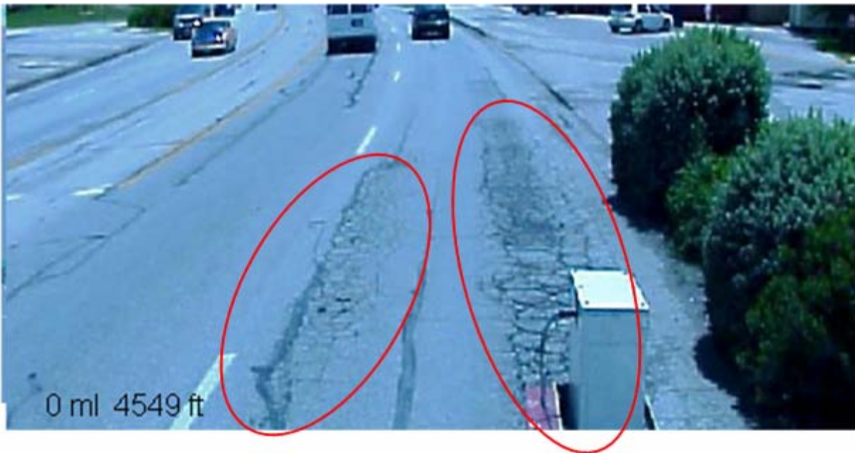
Figure 7-2. Wheel Path Surface Cracking on US 281 (Marble Falls) – Southbound Lane.
