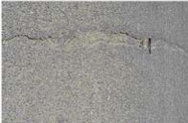
Figure 2-1. Example of Cracking Greater than 0.25 inch – Seal Prior to Overlay.
