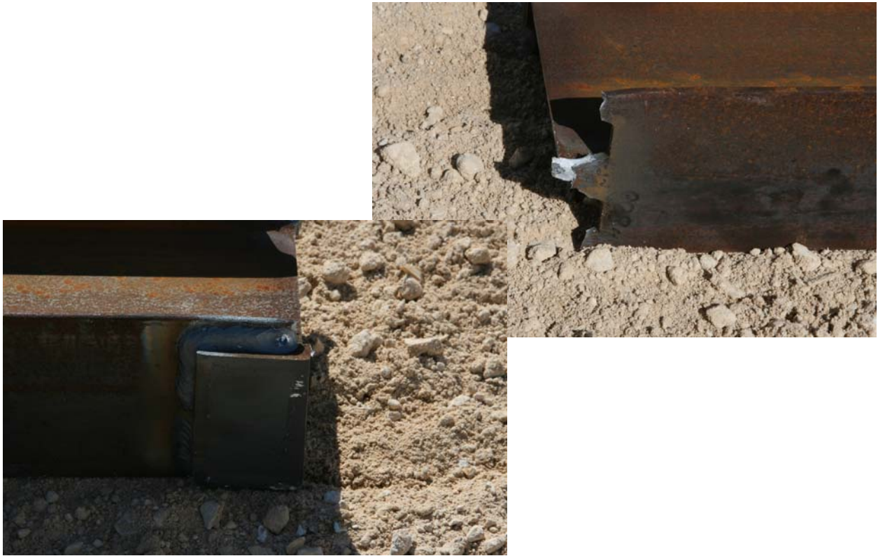
Figure 4.4. T8 Post with 7/8-Inch Slots after Test 452107-P1.
