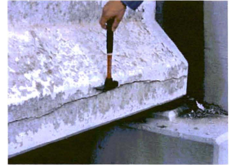
Prestressed concrete beam with Premature Concrete Deterioration
