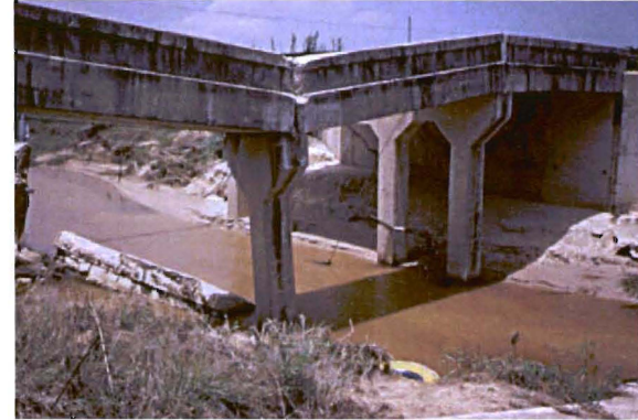
Scour of soil from around bridge piers can ultimately lead to structural failure
