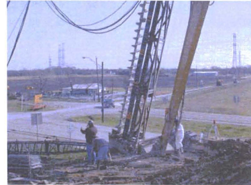
CFA pile installation for bridge foundation at Krenek Road and US 290 in Houston.
