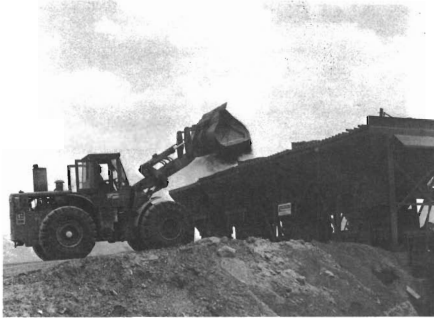
Figure 27. Front-end loader fills the three bins that are being used for this project.
