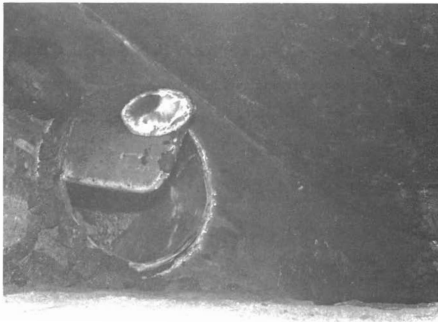
Figure 37. Interior view of the portal in which the fine particle return line feeds the particles back into the dryer drum.
