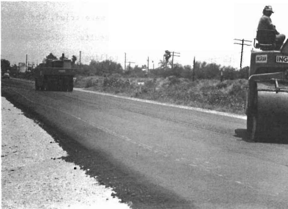
Figure 48. Rubber tired rollers followed the steel flat wheel roller for final compaction.
