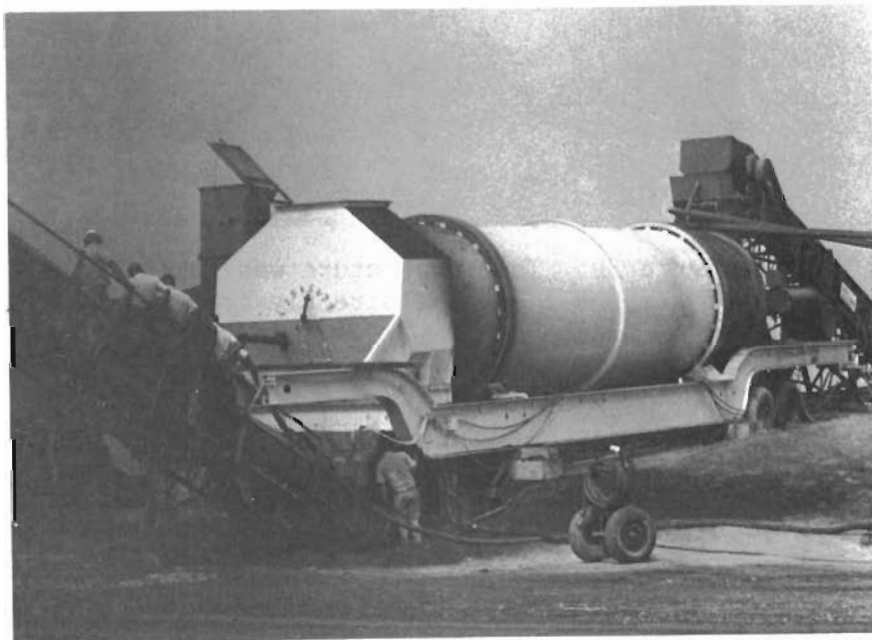
Figure 32. Time: 10:47 a.m. - Plant has been readjusted, the plume barely visible, so the various experts are examining the finished recycled hot mixed asphalt.
