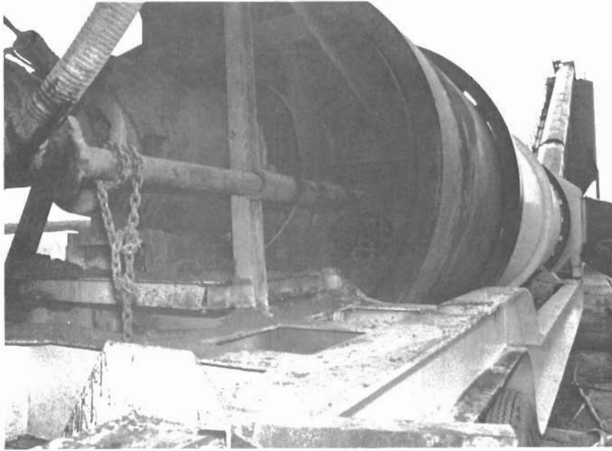
Figure 13. The modified end of the dryer drum shows the ceramic grid thru the port holes. Flexible pipe line connects to pipe feed to the dryer drum.
