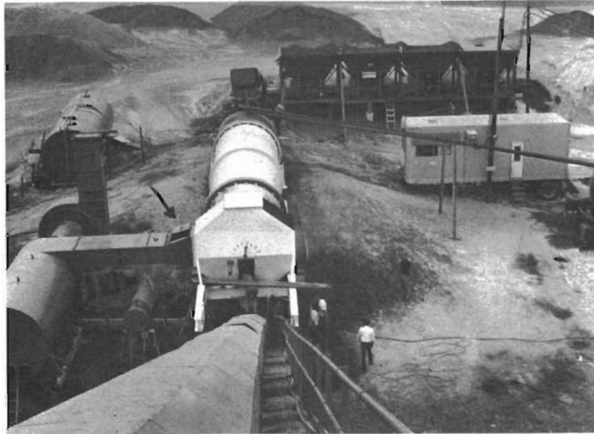
Figure 21. Overview from top of the hot-mixed storage bin looking at the plant while it was being repaired. The dust collector line has been reinstalled below the frame of the dryer-drum frame.
