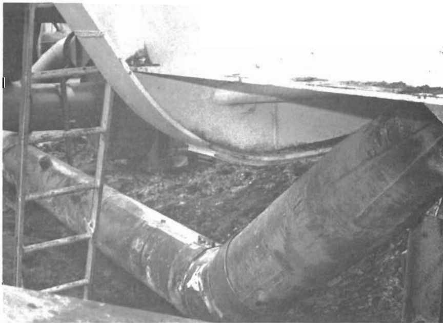
Figure 38. The completed modified return line for the fine particles from the dust collector.
