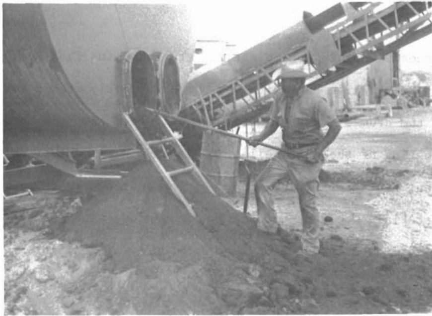
Figure 29. East end of dust collector. Excessive dust was collected which was not returned to the dryer drum, resulting in a required modification of plant.
