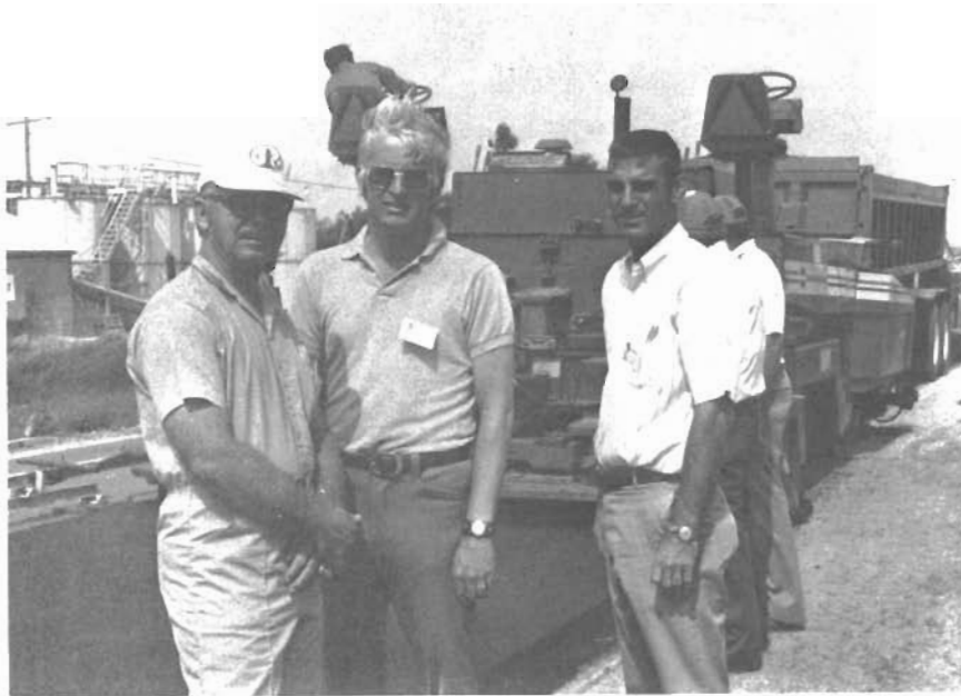
Figure 8. Charles Hughes, Tom Kennedy and Jon Epps observe the lay down of the recycled HMA.
