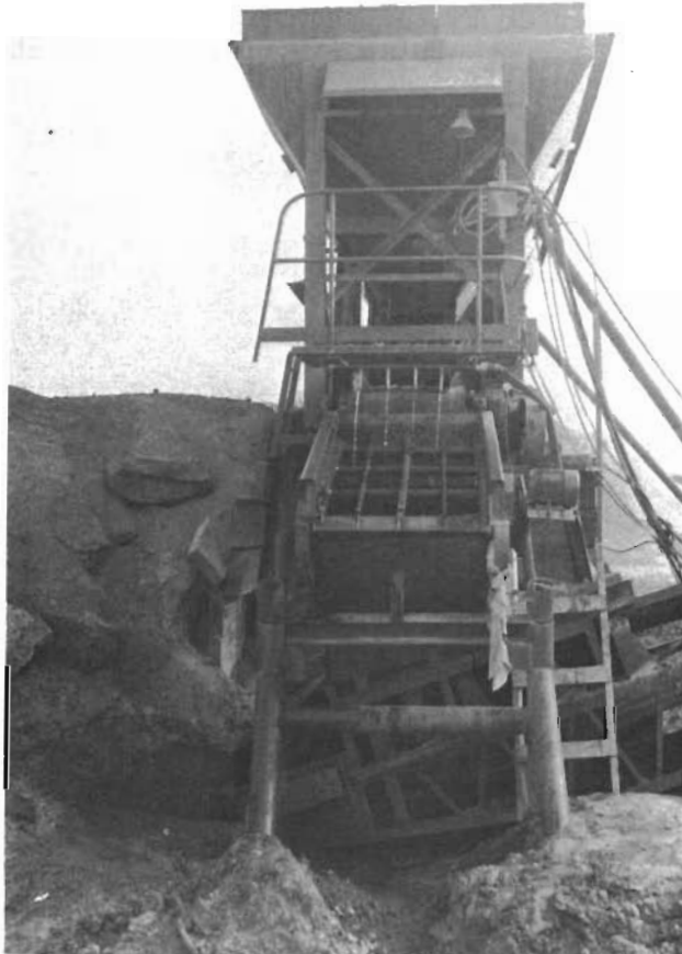
Figure 18. The control box for change of direction of flow of material on conveyor belts.
