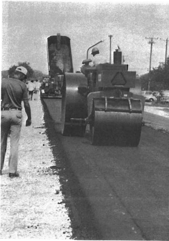
Figure 47. Steel flat wheel rollers followed the lay-down machine as closely as possible to get good compaction.
