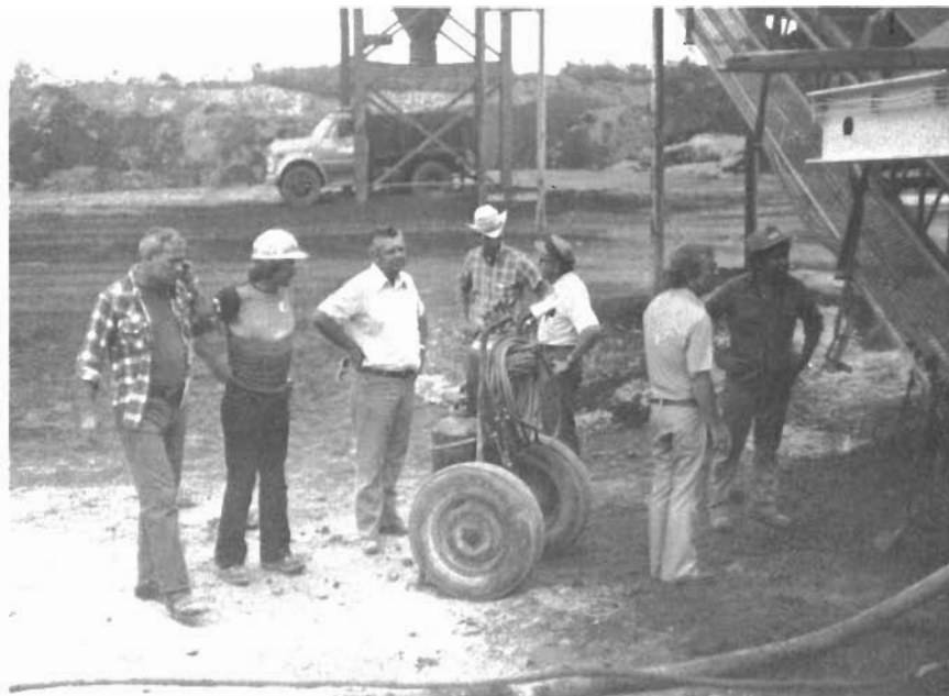
Figure 9. Douglas Bernard, Steve Beckett, Harry Goss, Sim Giles, Arthur Hill, Chuck Looney, and M. Israel observe modification during the welding of a new opening for the return dust line to the dryer drum.
