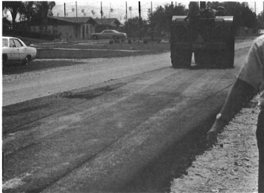
Figure 44. Flat wheel rollers were used first in the compaction of the hot mixed asphalt overlay.
