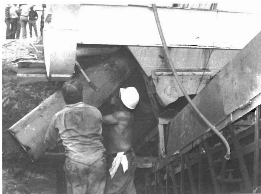
Figure 36. The fine particle lines were lowered below the dryer drum frame to give a better mixing of the fines with the rest of the out-flow of hot mixed asphalt.
