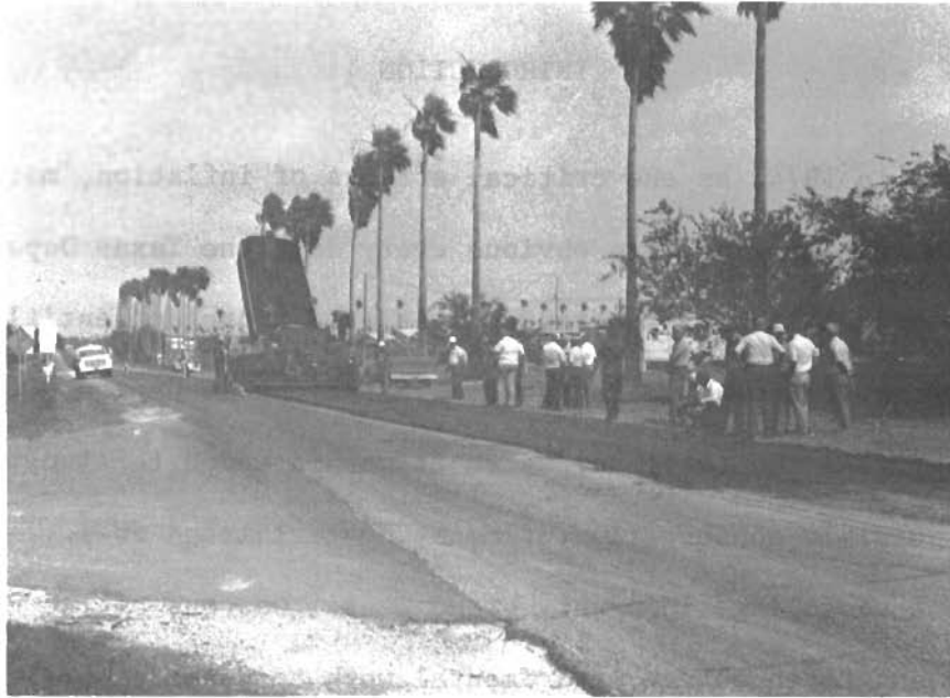
Figure 2. District 21 experimental hot mixed asphalt overlay project on Old U.S. 83, west of Mission, Texas. The project utilized recycled asphalt pavement and base material which was removed from N. 10th St. in McAllen, Texas.
