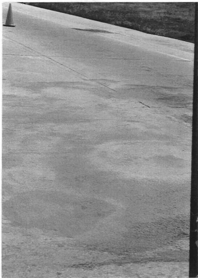
Figure 8. MMA-based polymer mortar repairs to failed PUP repairs in repair area 1 (slabs 11 and 12).
