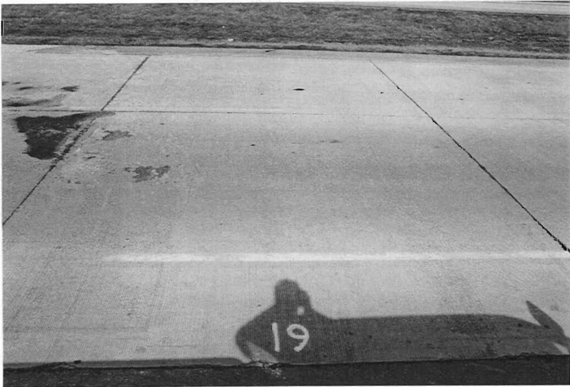
Figure A-11. Slab 19, like slab 18, has deeper spalls in the outside lanes and an area of light spalling on the inside lanes.
