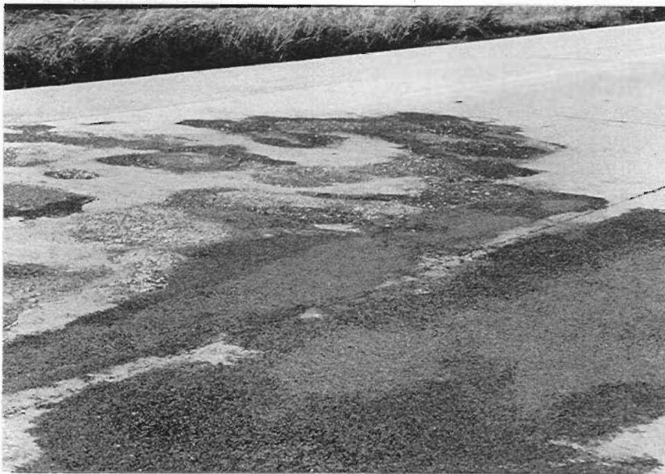
Figure 7. Area 5, consisting of slabs 41 and 42, shows that repairs were made of different materials. No significant deterioration has occurred.
