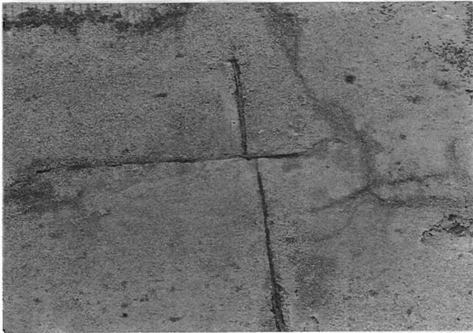
Figure 10. Detail of cardboard inclusions in MMA mortar for stress relief over substrate joints shows little deterioration.
