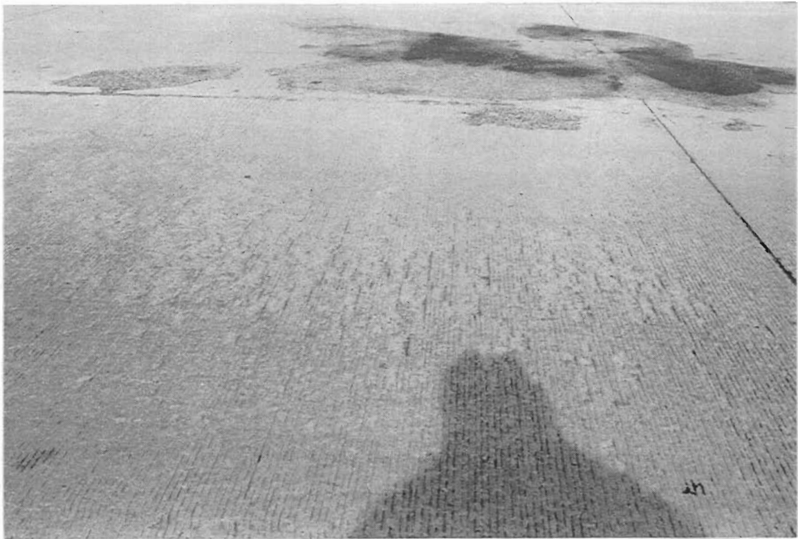
Figure A-3. Slab 11 shows light surface spalling in the foreground and asphalt filling the deeper spalls in the background.
