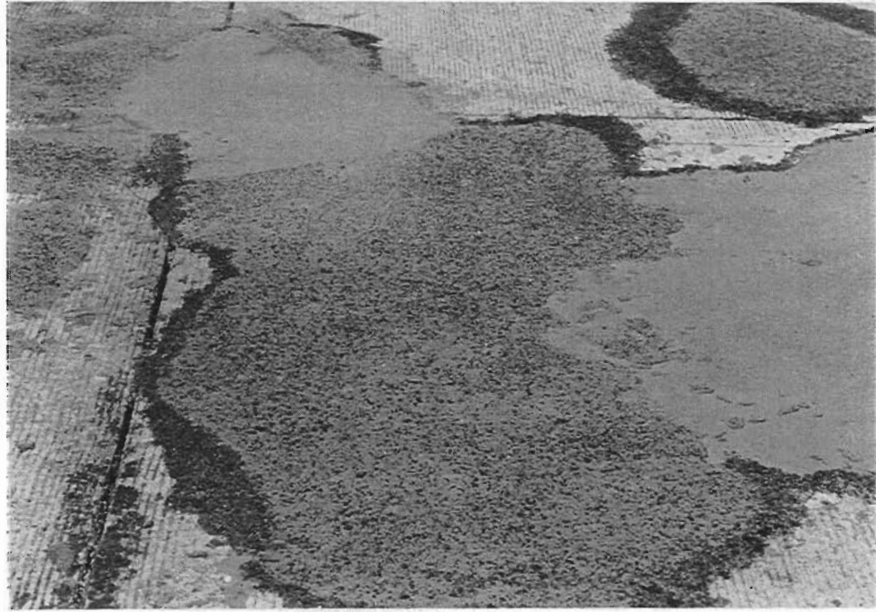
Figure 11. PUP mortar in repair area 2 (slabs 14 and 15) is still in good condition after one year.
