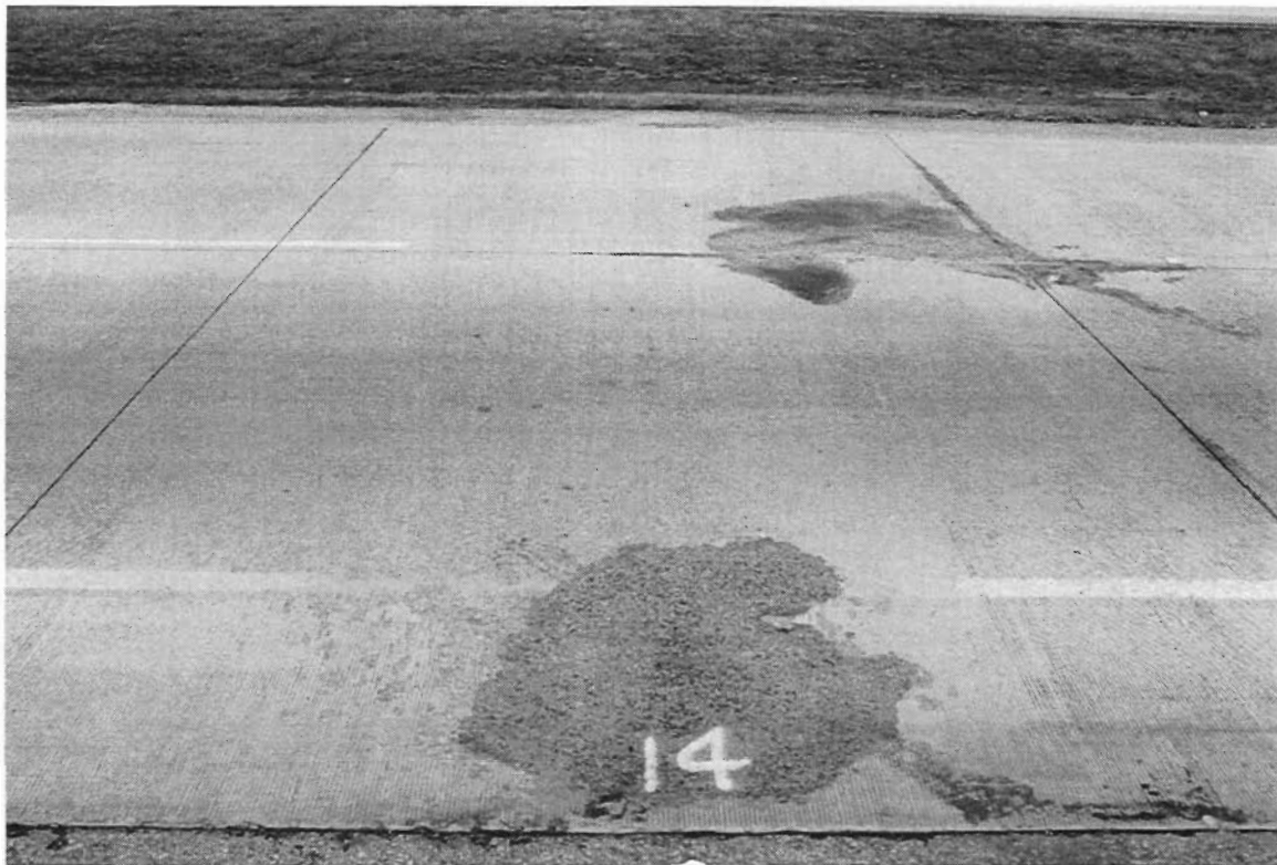
Figure A-6. Slab 14 shows asphalt-filled spalls in both outside and inside lanes.
