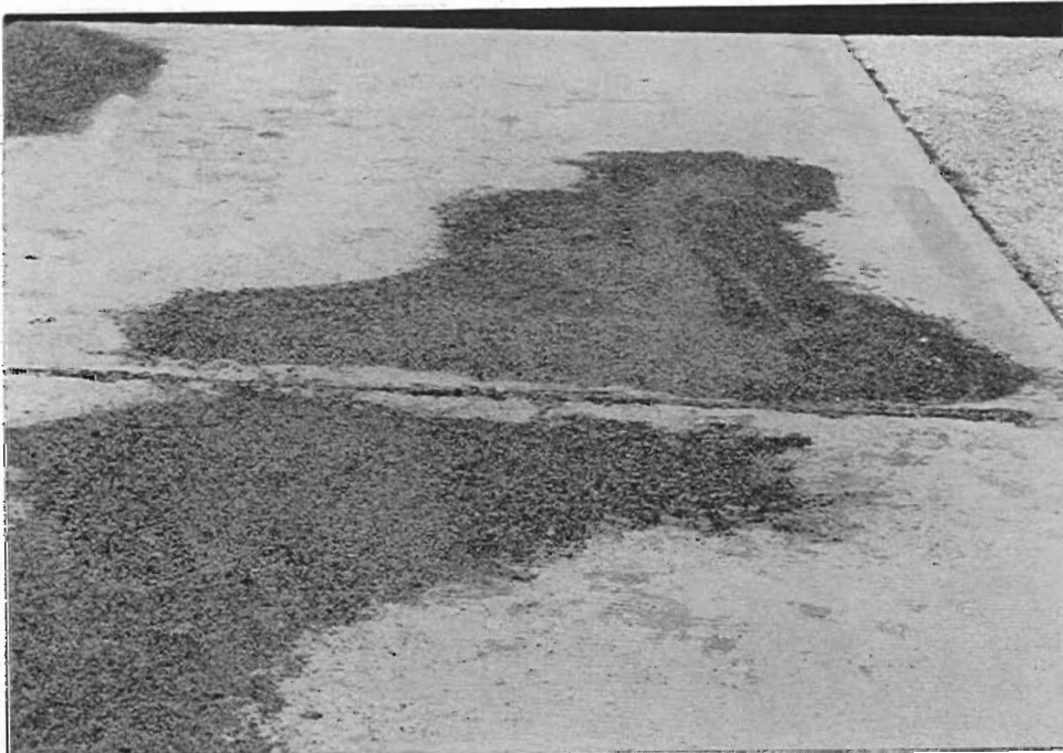
Figure 5. Area 3, consisting of slabs 18 and 19, still appears to be in good condition.
