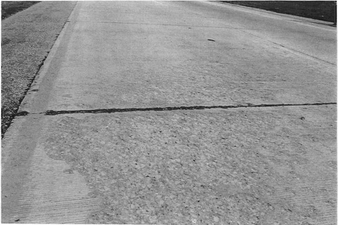
Figure A-10. An area of light spalling is also apparent on the inside lanes of slab 18.
