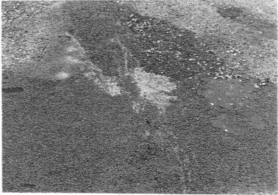
Figure 15. Some reflective cracking from substrate through epoxy mortar has occurred at one year.
