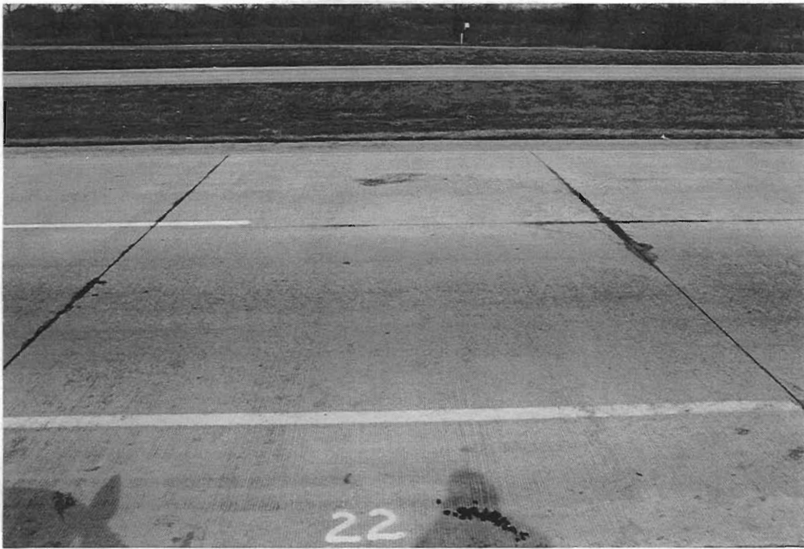
Figure A-13. Slab 22 shows one deeper spall in the middle of the inside lanes and another along the transverse joint with an area of light spalling between the two.
