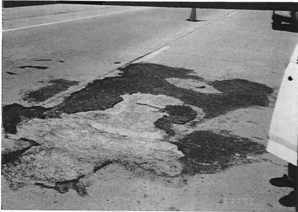
Figure 2. Repair area 1, consisting of the repairs to slabs 11 and 12, shows large areas of delaminated and broken chunks of PUP material.
