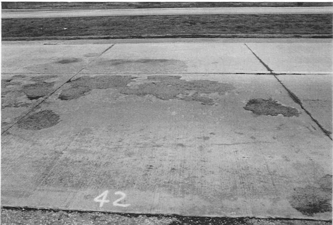
Figure A-17. Slab 42 shows a few areas of deeper spalling surrounded by a large area of light surface spalls.
