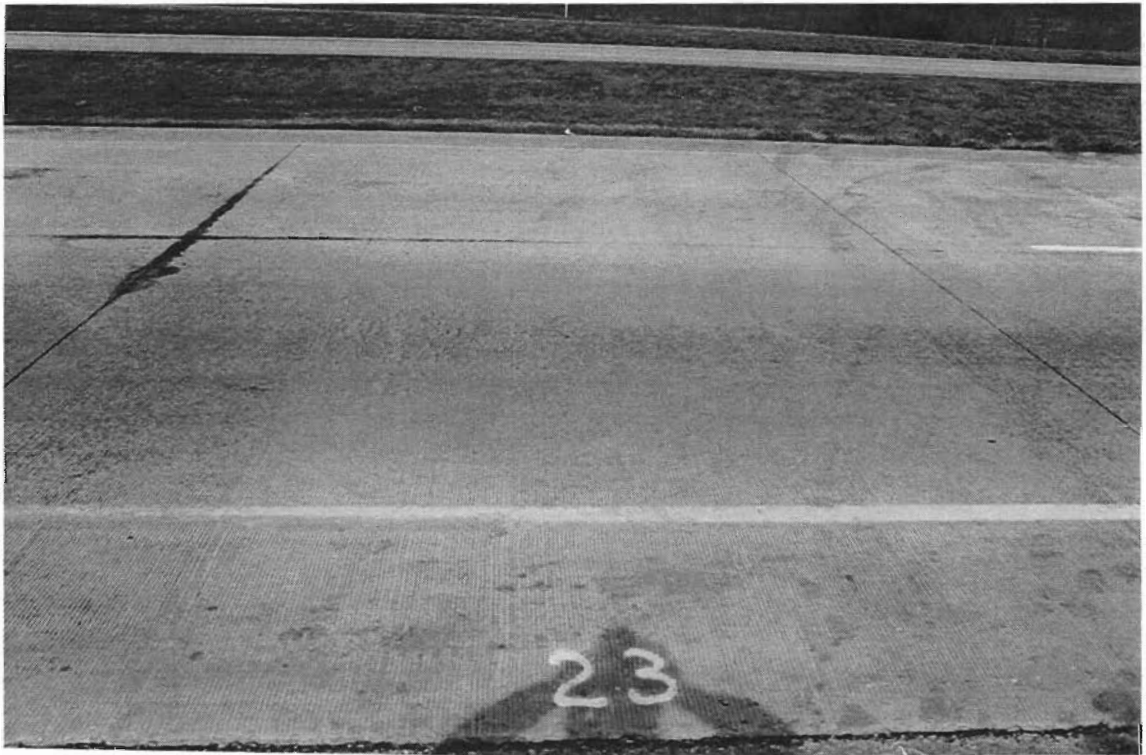
Figure A-14. Slab 23 has a small area of light spalling adjacent to the deeper spalling at the transverse joint.
