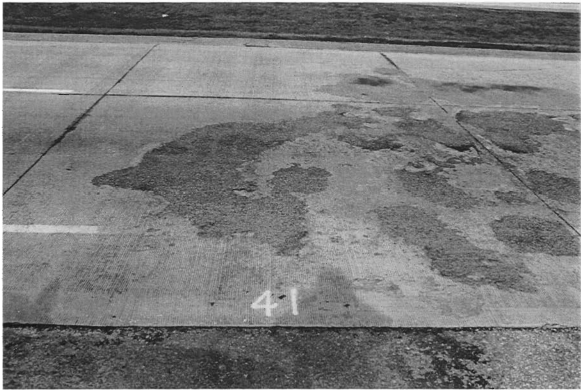
Figure A-16. Slab 41 shows several large areas of deeper spalling.
