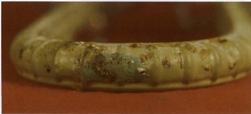
Figure 3.1 Corrosion of patched area of #4 epoxy-coated bar (macrocell study).
