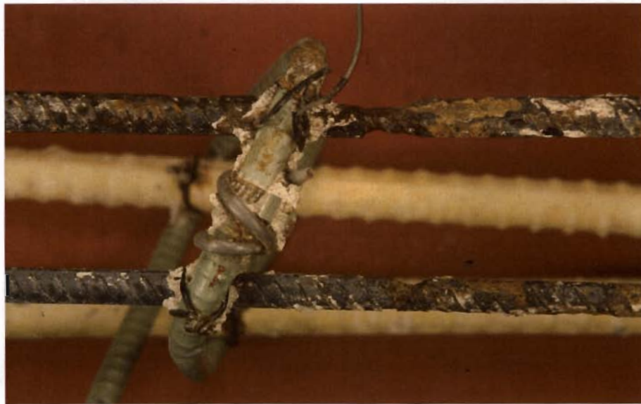
(b) Severe pitting on black bars near coated stirrup (beam B23).
