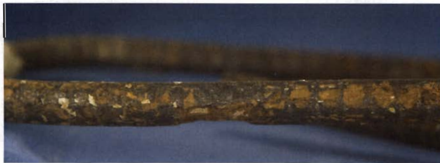
Figure 2.18 Pitting along stirrup leg surface beneath the coating (beam B27).
