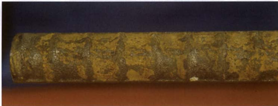
Figure 3.5 Underfilm corrosion of splice bar after 4.3 years of exposure (beam study).
