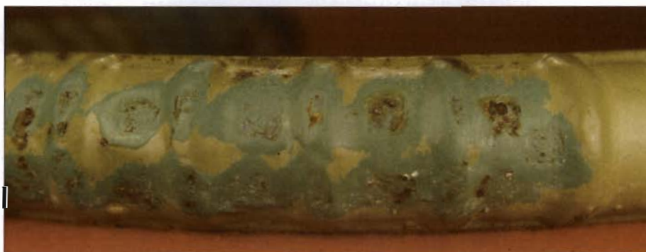
Figure 2.10 Corrosion of patched areas at outside bend on #8 bar with damaged coating greater than 2%.
