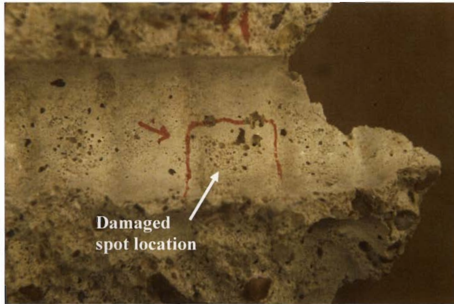
Figure 4.2 Concrete surrounding uncorroded damaged spot within the wetted region (Upper bar of beam B10).
