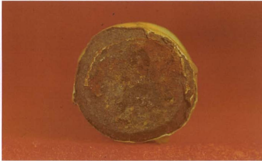
Figure 3.11 Corrosion of bar end surface that was specially cleaned before patch application.
