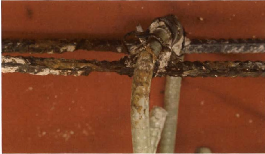
(a) Severe pitting on lower black bar near coated stirrup (beam B23).
