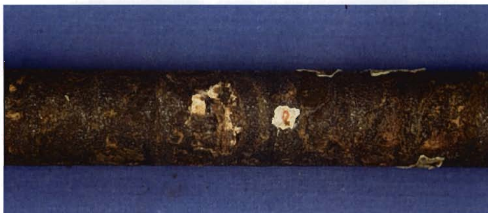
Figure 3.19 Dark corroded surface beneath debonded coating on longitudinal bar with 3% damaged coating within the wetted region (beam B8).
