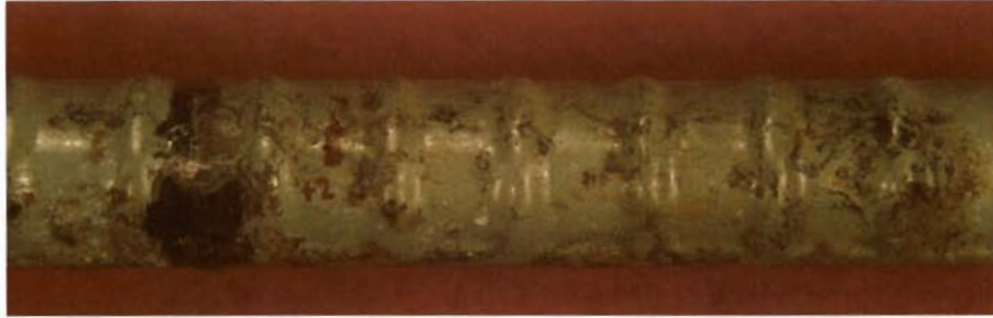
(a) Rust stains at lower bar of beam B10, portion within the wetted zone. Damaged spot at crack location.
