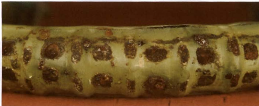
Figure 2.9 Corrosion of damaged areas at outside bend on #8 bar with damaged coating greater than 2%.
