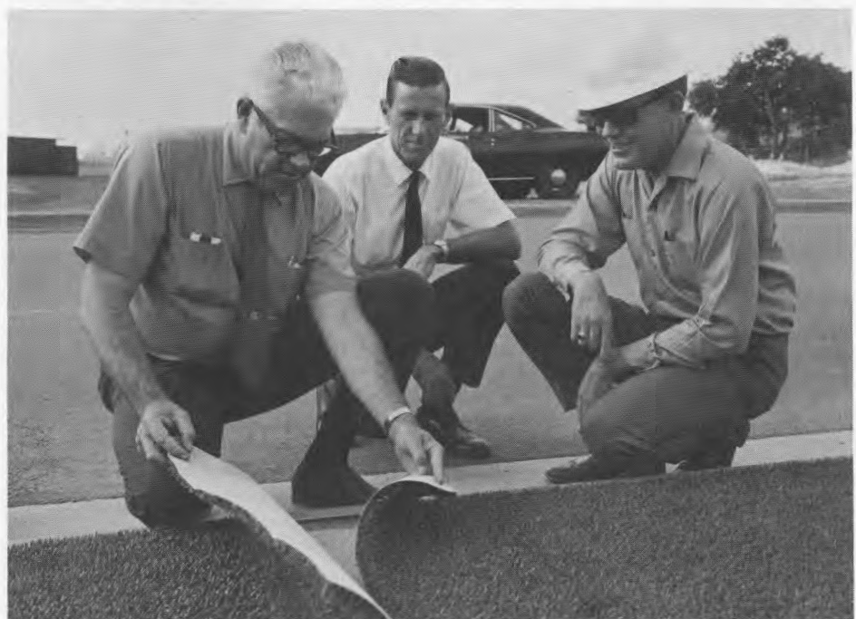
A SPECIAL landscaping surface of AstroTurf, the wonder fabric of the synthetic world, is being tested on a median in Austin. Time will tell about its durability. If it stands up well this year, the Highway Department may install AstroTurf on other medians and traffic islands. The test section, being inspected by Clarence Rea and Bob Reed of Bridge Division and District 14's Ben Alley, is on RM 2222, part of Austin's Mo Pac Expressway project.
