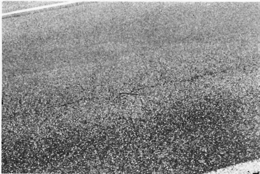
(NO WIRE REINFORCEMENTS)
