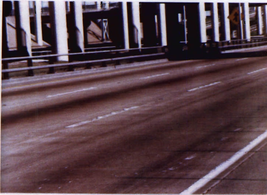
Figure 15: 1977 Test Section of Stud Bottom Oval Markers. Note Maintenance Forces have striped over the Markers. Picture taken on 1-26-87
