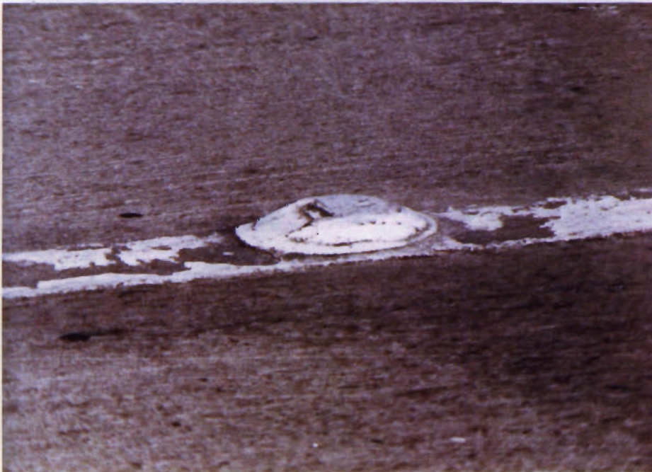
Figure 16: Ten Year old Marker in the 1977 Test Section. Note REFLECTIVE Rod is Missing. Picture taken on 1-26-87
