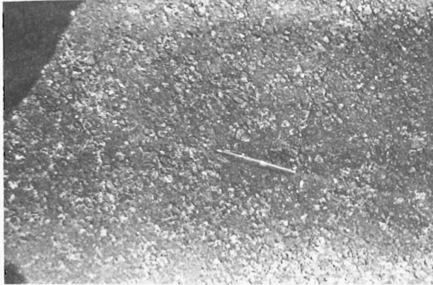
Sprinkled Section Type "F", grade 4 Synthetic Rolled into the Type "D" ACP
