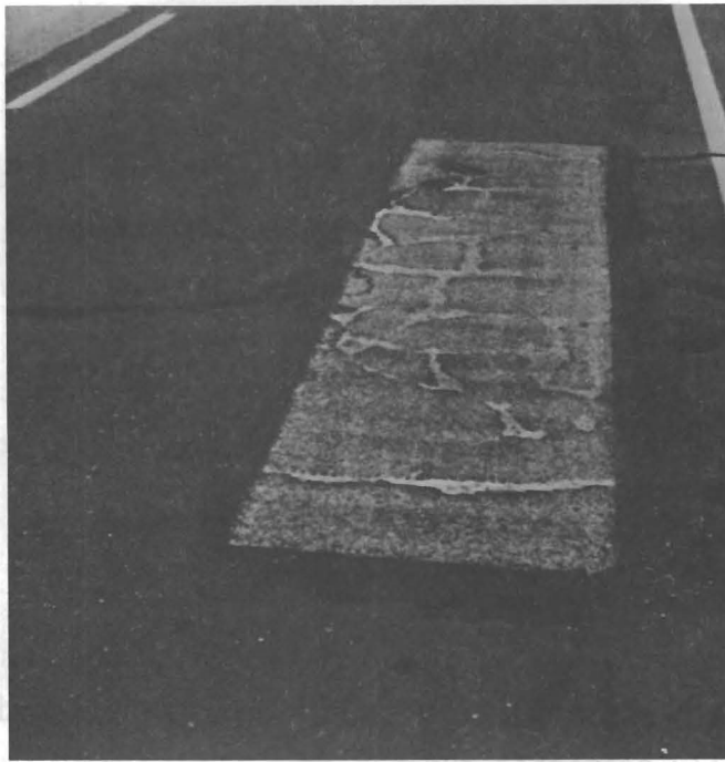
Patch in Place 1½ Years
