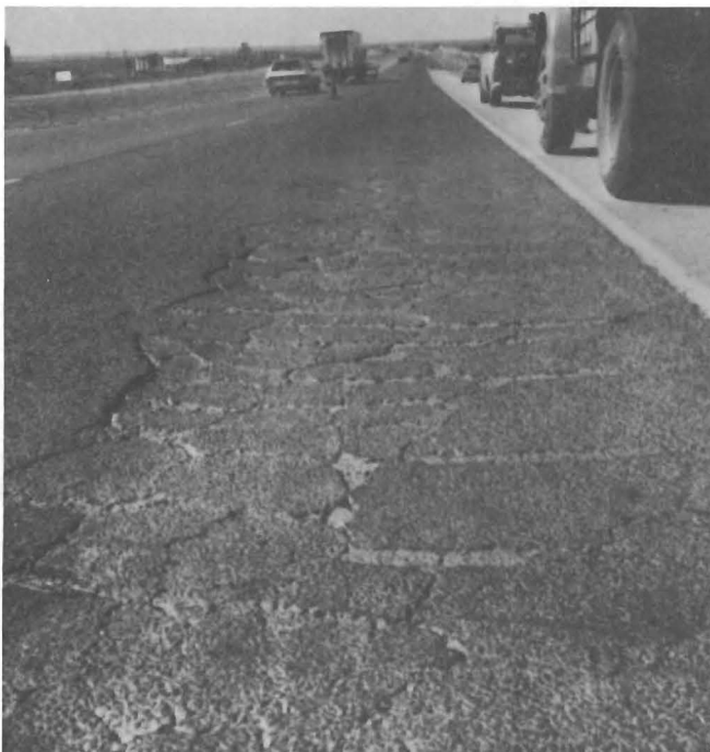
Badly Alligatored Pavement
