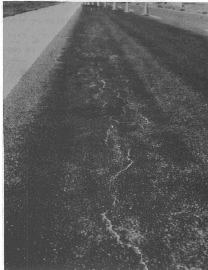
Typical Cracks To Be Repaired
