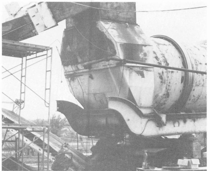
6. Rear of drum showing asphalt line and latex nozzle assembly guide tube
