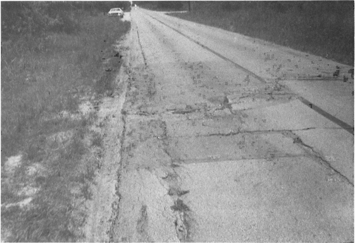
Figure 1: Condition of roadway prior to treatment
