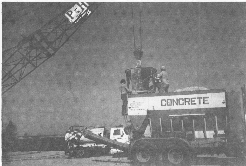
Figure 10. Mobile Concrete Batch Truck
