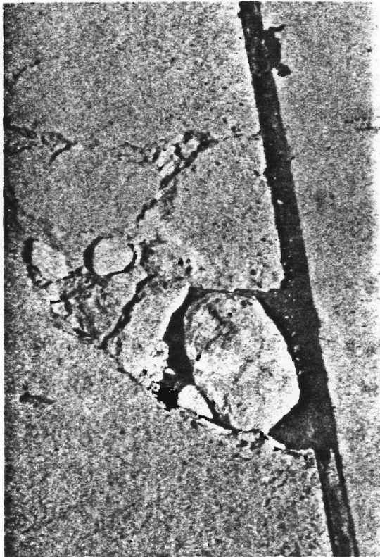
Figure 1 - Damaged Area of Concrete Pavement
