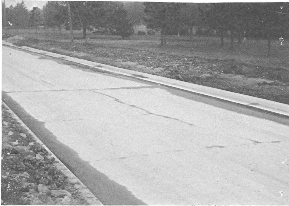
Lateral and longitudinal cracks in second course of expansive cement stabilized base.
