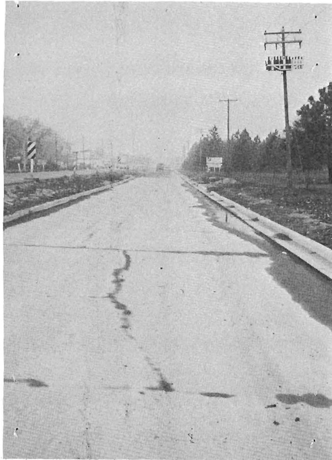
Lateral and longitudinal cracks in second course of expansive cement stabilized base.
