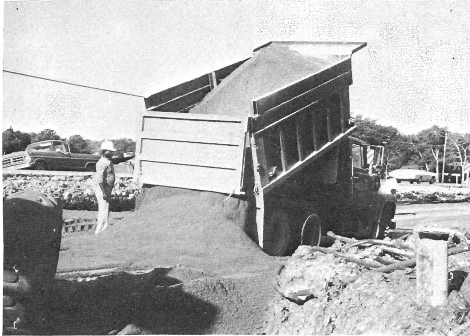
Placing cement stabilized gravel screenings base on untreated subgrade.(TXI 4C Chem Comp expansive cement test section)
