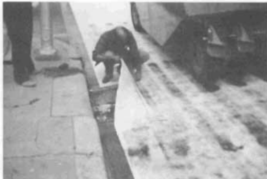
PORTIONS OF FABRIC OVER INLETS, MANHOLES AND VALVES WAS EASILY CUT WITH POCKET KNIVES AND REMOVED.
