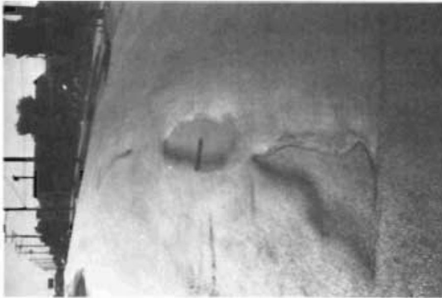
-PHOTO 34-79A- LONGITUDINAL SHOT EASTBOUND LANES AT BEGINNING OF PROJECT. VICINITY OF SLIPPAGE AREA NO. 1.
