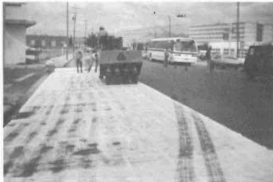
FABRIC UNDERSEAL PLACEMENT PROCEDURES INCLUDED TWO PASSES OF A MEDIUM WEIGHT PNEUMATIC TIRE ROLLER.
