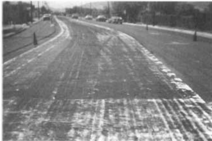
APPEARANCE OF FABRIC UNDERSEAL ON A CURVE AFTER COMPLETION OF TWO PASSES OF A MEDIUM WEIGHT PNEUMATIC TIRE ROLLER AND AWAITING THE A.C. PAVEMENT OVERLAY.
