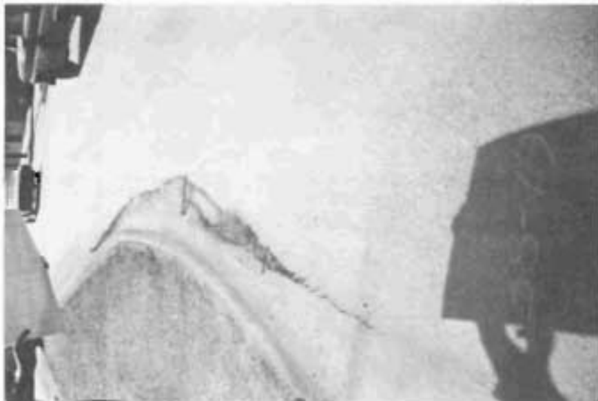
-PHOTO 38-79- SLIPPAGE AREA NO. 1 - STATION 164 + 60 ±
