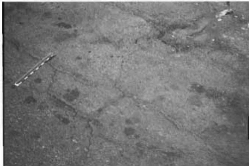
PHOTO SHOWING TYPICAL POTHOLES WHICH EXISTED MOSTLY ALONG CURB.
