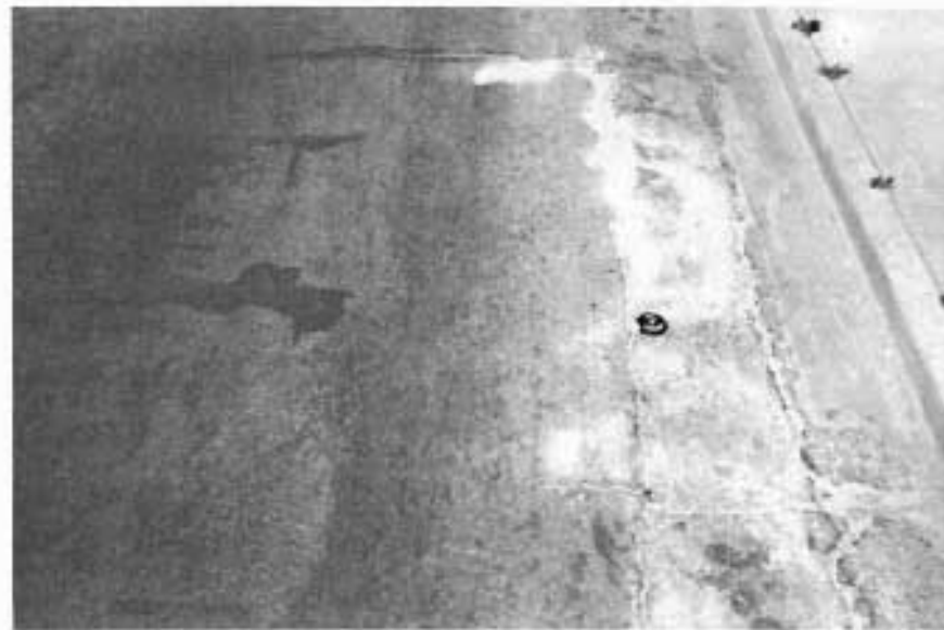
THIS PHOTO DEPICTS ONE OF SEVERAL UTILITY CUTS THAT EXISTED WITHIN THE LIMITS OF THIS PROJECT.
