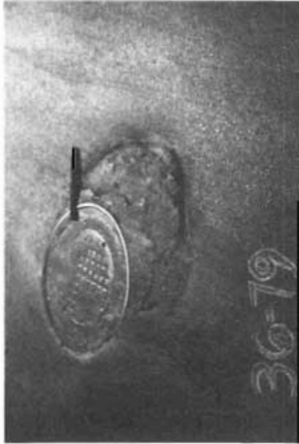
CLOSE-UP OF PAVEMENT SLIPPAGE AT MANHOLE... EASTBOUND LANES AT BEGINNING OF PROJECT. VICINITY OF SLIPPAGE AREA NO. 1.
