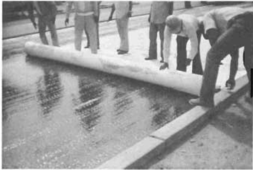
PLACEMENT PROCEDURES INCLUDED MAINTAINING APPROXIMATELY 3" BETWEEN FACE OF CURB AND EDGE OF FABRIC.
