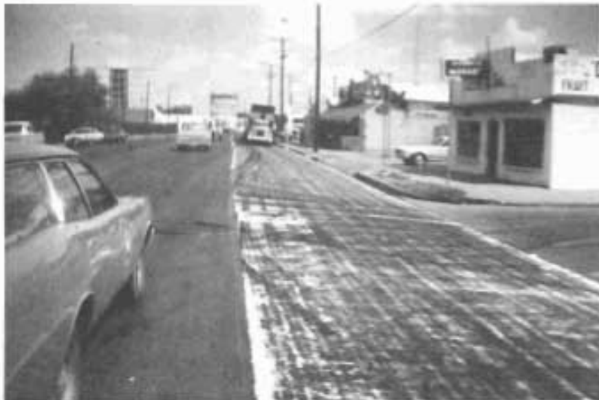
PLACEMENT OF THE FINISH A.C. PAVEMENT OVERLAY WAS IN PROGRESS SHORTLY AFTER FABRIC WAS PUT DOWN.
