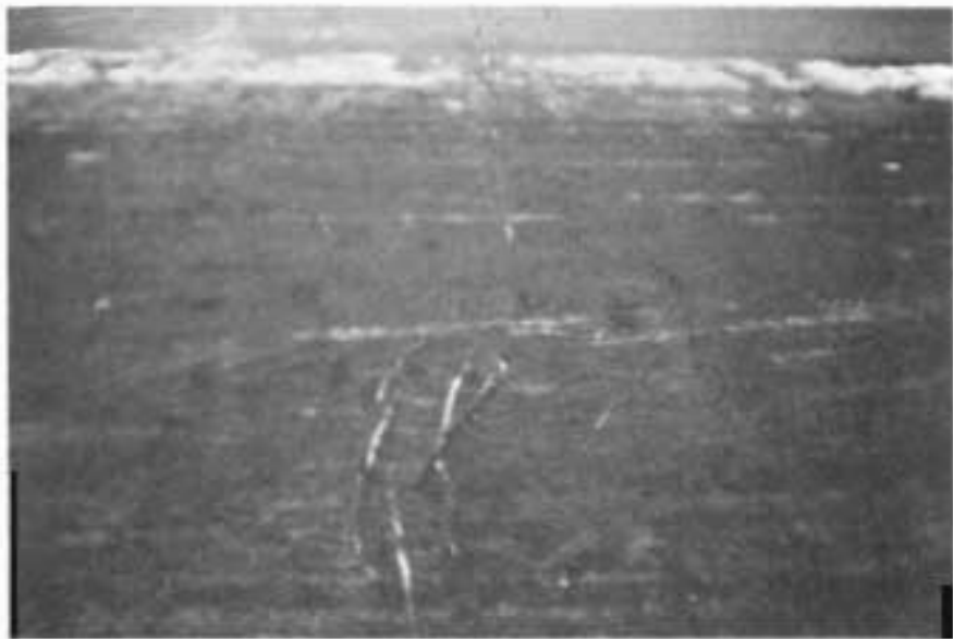
APPEARANCE OF FABRIC UNDERSEAL AFTER COMPLETION OF TWO PASSES OF A MEDIUM WEIGHT PNEUMATIC TIRE ROLLER, BUT WITH NOTICEABLY MORE ABSORPTION OF AC-10 THAN IN SOME OTHER PLACES.
