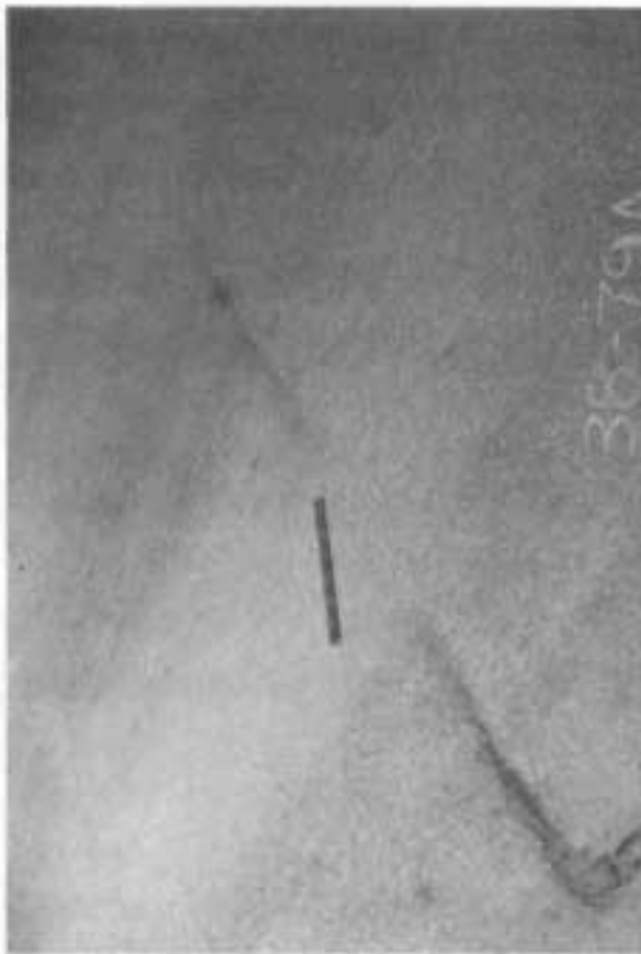
- TRANSVERSE CRACK- AT EASTERN END OF LONGITUDINAL CRACK OF SLIPPAGE AREA NO. 1.
