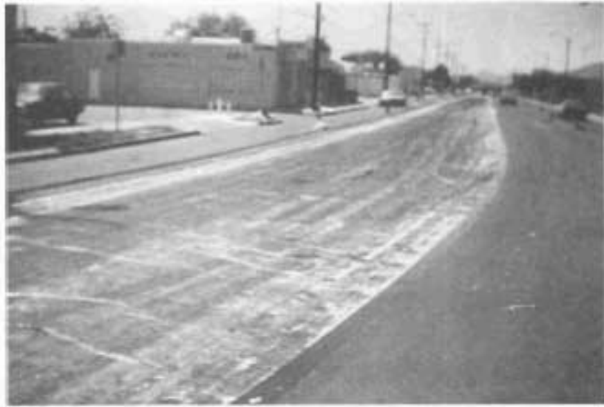
ANOTHER VIEW OF THE SECTION IN THE PHOTO BELOW BUT REVEALING MORE PRONOUNCEDLY THE TYPICAL WRINKLING.
