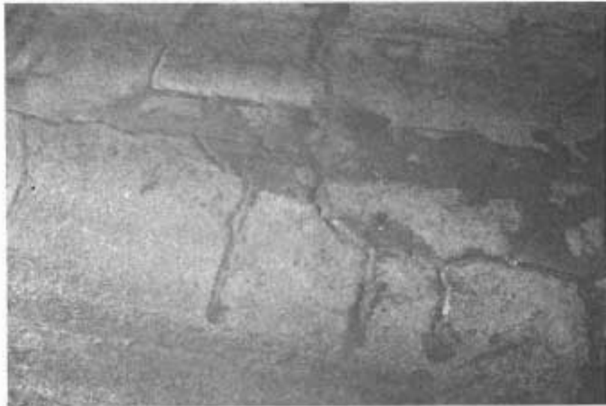
PHOTO DEPICTING CRAZED PATTERN OF CRACKS; EVIDENCE OF BEING SEALED; AND RECRACKING.
