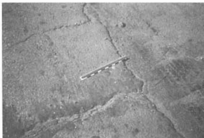
PHOTO DEPICTING BOTH LONGITUDINAL AND TRANSVERSE CRACKING. THIS LOCATION WAS APPROXIMATELY IN THE CENTER OF OUTSIDE WESTBOUND LANE.
