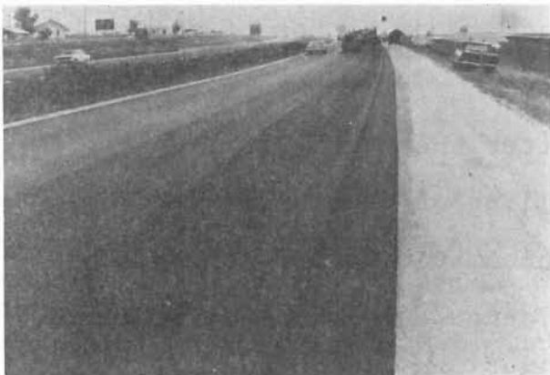
Rolling With Three Wheeled Roller Continues To Be Followed By Tandem Roller
