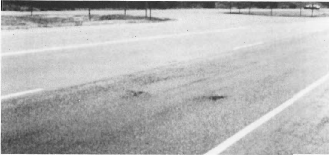
Figure 11.5. Spot segregation due to emptying hopper wings.
