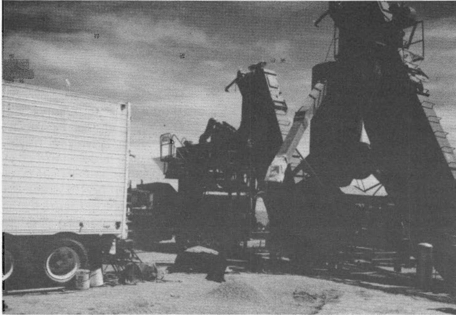
Figure 1.3. A typical continuous mix plant.
