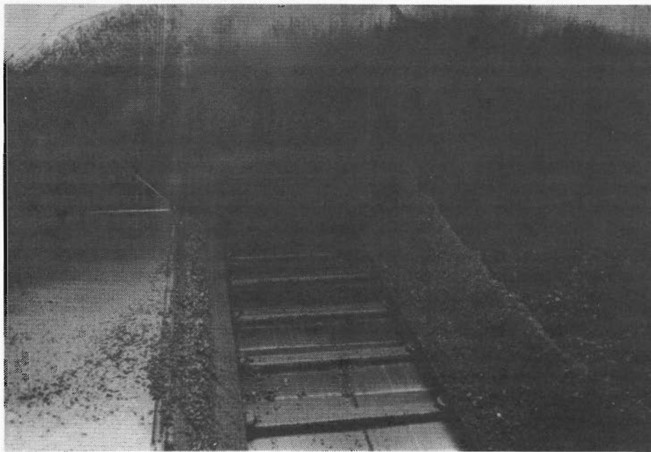
Figure 12.6. Flow gates in lowered position.
