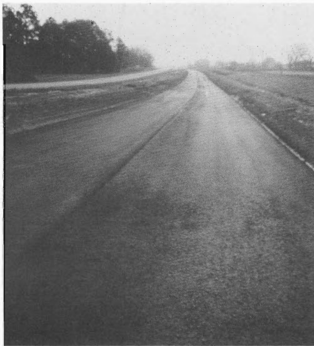
Figure 11.4. Systematic spot segregation between truckloads.
