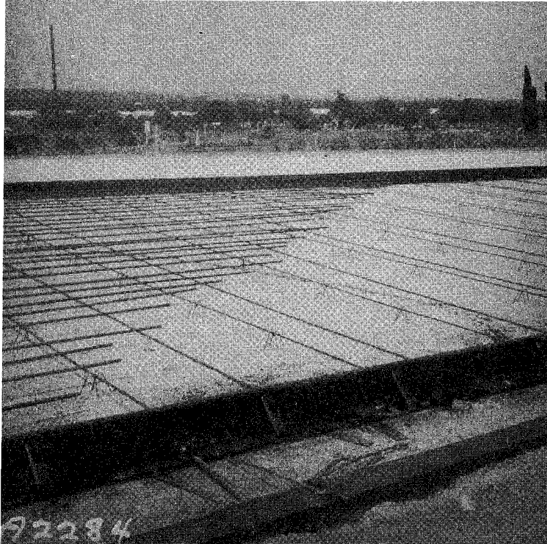
FIGURE 13: VIEW OF THE REINFORCING STEEL FOR CONTINUOUSLY REINFORCED CONCRETE PAVEMENT SHOWING THE STAGGERED BAR LAP
