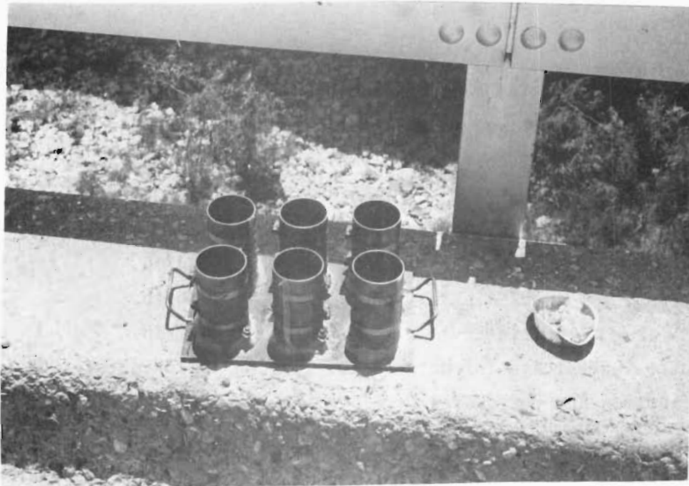
DAMAGED CONCRETE IN CURB FROM CHEMICALS AND FREEZE THAW
