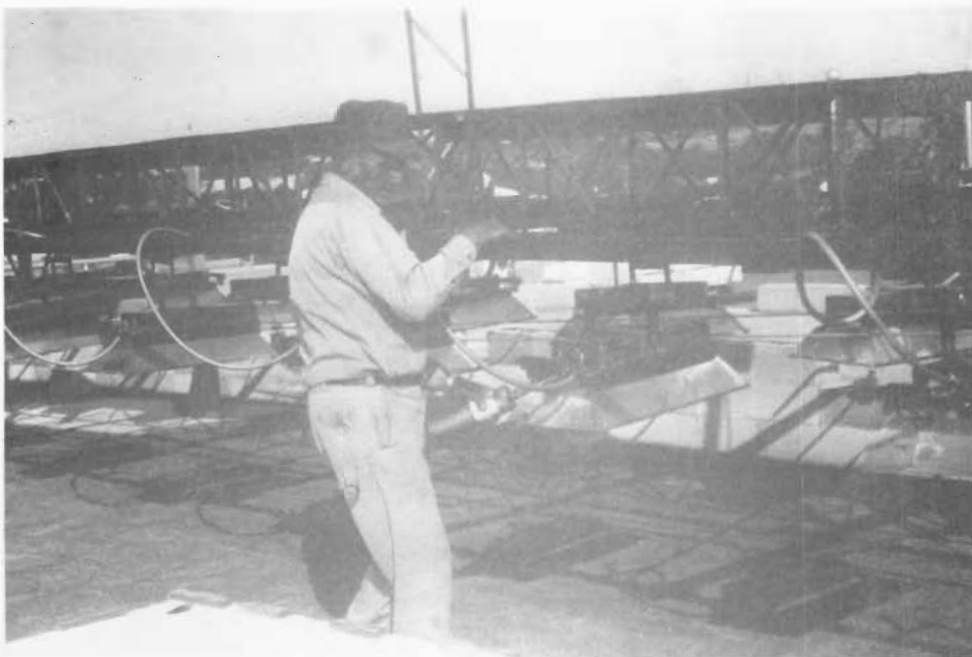
LIGHTING THE RADIANT HEATERS
