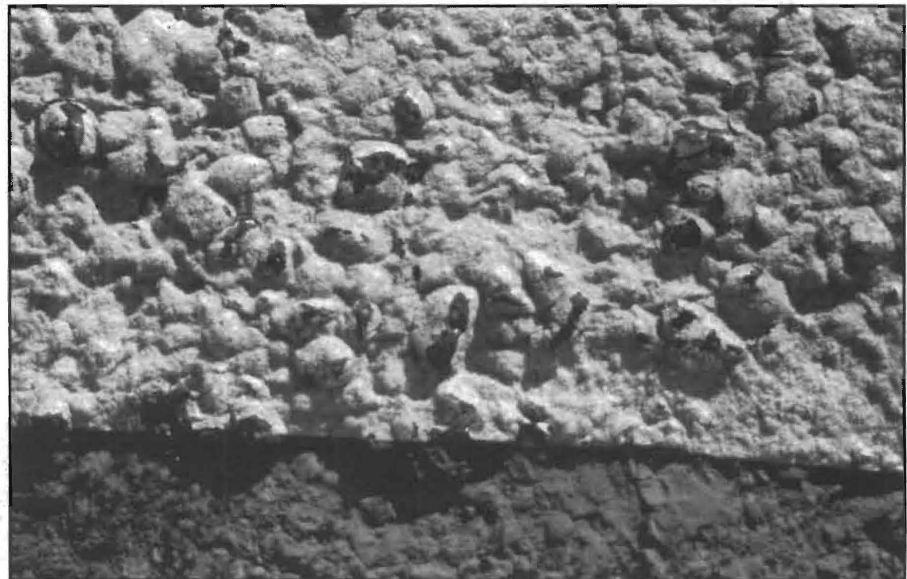
FIG. 2: Although gravel has punched through the tape in places, the retroreflectivity is still well above minimum
