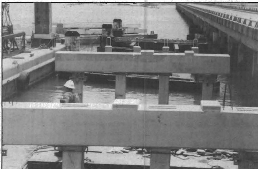
FIG. 5: Completed interior bents. Note pile tops in background ready for precast bent cap placement.
