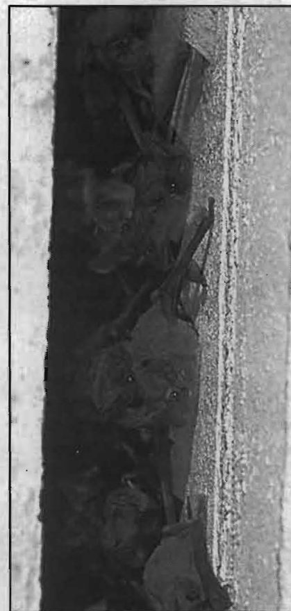
FIG. 2: Mexican free-tailed bats roosting between beams in Congress Avenue Bridge. Any vertical crevice in concrete, from 3/4 inch to 1-1/2 inches wide by 12 inches or more deep is likely to attract bats. Vertical holes 2 to 6 inches in diameter and 12 to 24 inches deep simply attract different kinds of bats. The deepest holes or crevices are best.
