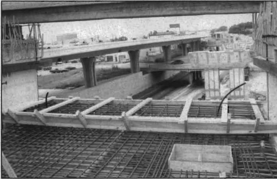
FIGURE 2: The "Y" was erected above existing travel lanes in very limited ROW. Construction innovations (like varying the width of the closure pour to keep transition boxes of a uniform size, shown here) reduced the overall cost.
