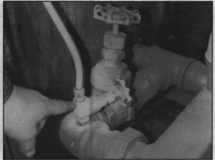
FIGURE 7: Diesel valve (white) — used when flushing system
