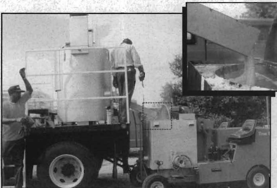
FIGURE 1: Thermoplastic is melted and transferred to the placement vehicle of the US 183 job.
