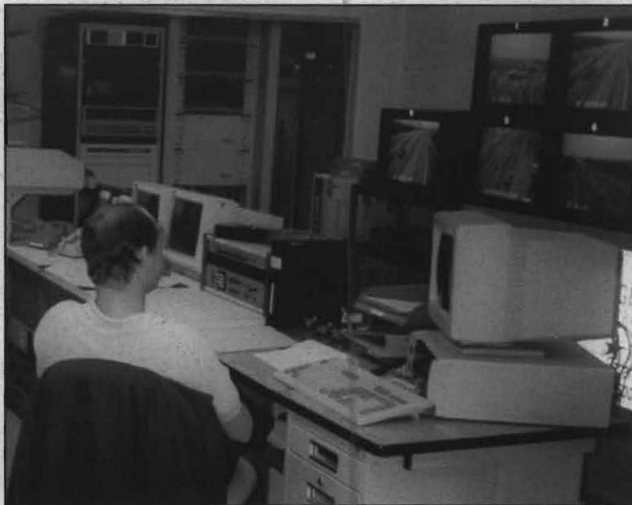
FIGURE 2: Monitoring traffic at the new control center.
