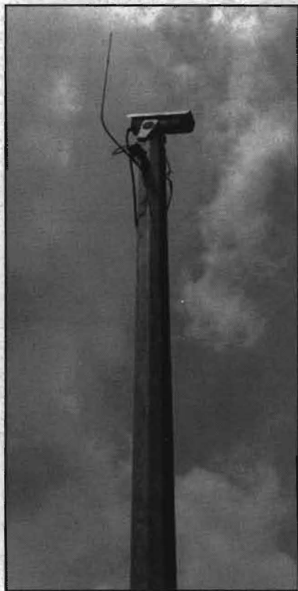
FIGURE 1: Closed-circuit TV camera in Fort Worth District.
